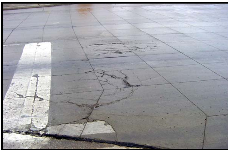
Figure 14 Bonded Concrete Area of Distress
