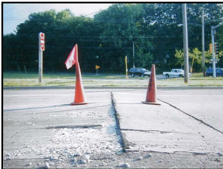
Figure 2 Bonded Concrete Inlay “Blow-Up” Failure
