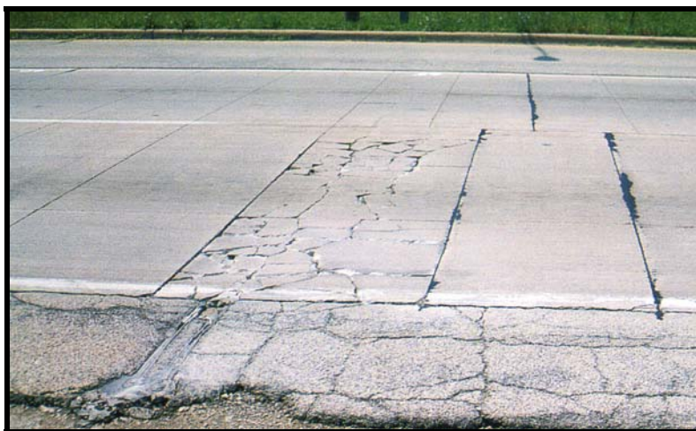
Figure 7 Distress at Traffic Indicator Loop
