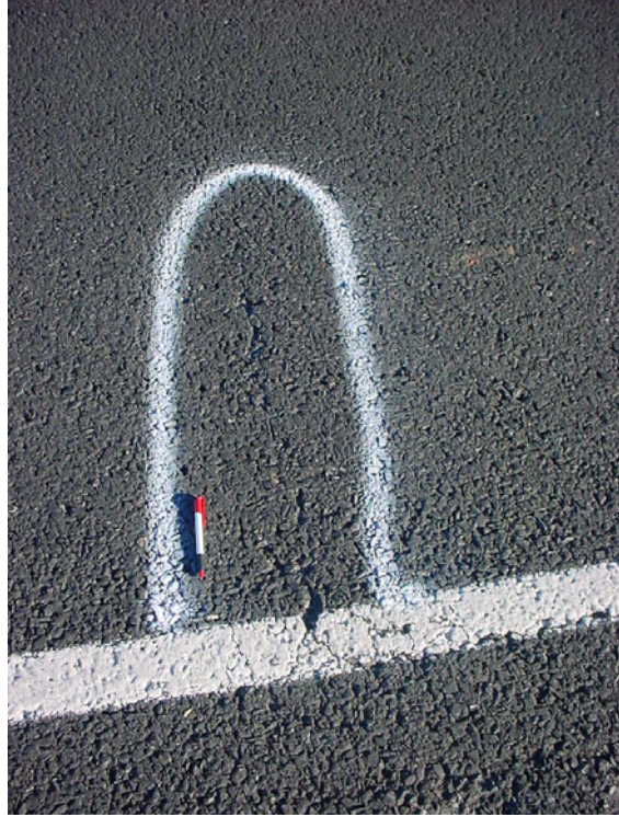
Figure 3.1 Low-level transverse crack
