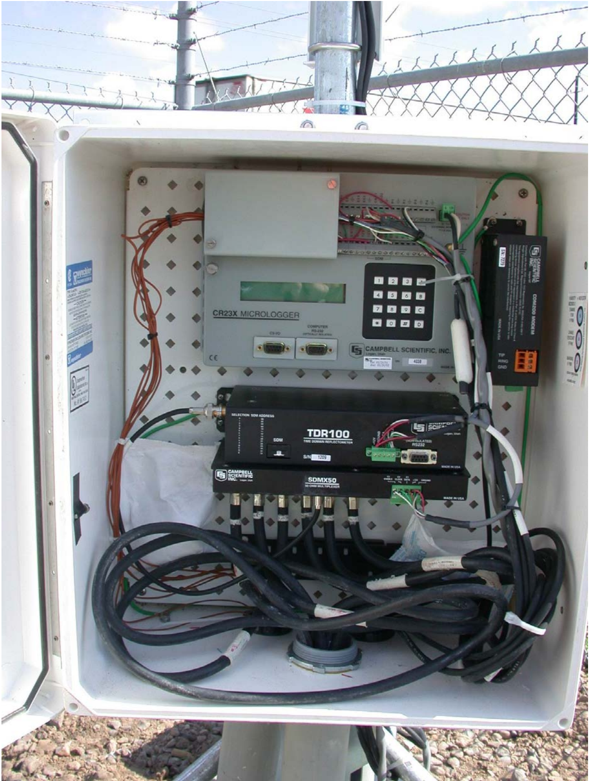
Figure B15. Weather Station Controller Box.
