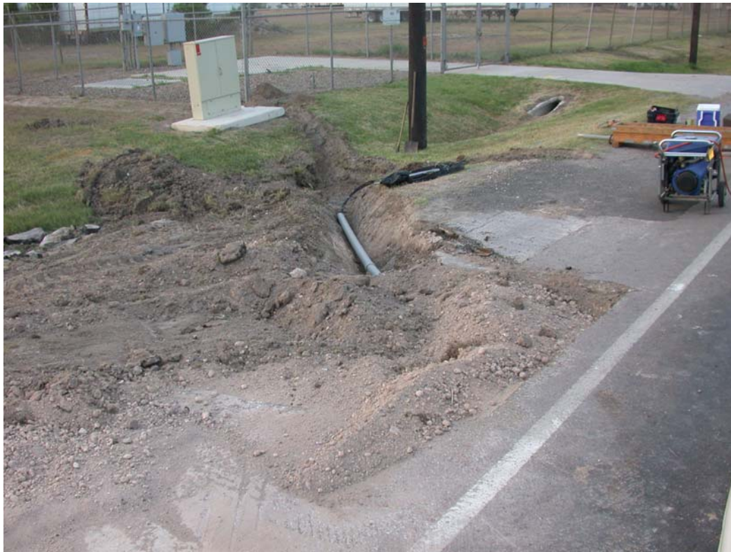
Figure B10. Sensor Cables Routed through a Conduit.
