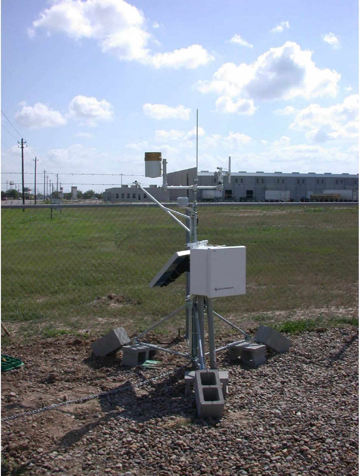
Figure B16. Weather Station Installed at WIM Site.
