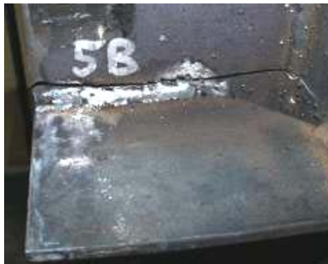
Figure 4-16: Crack at Toe of Weld 2T
