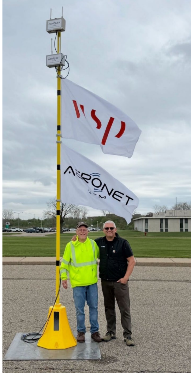
FIGURE 6. C-V2X AND DSRC RSU ON TEMPORARY POLE
