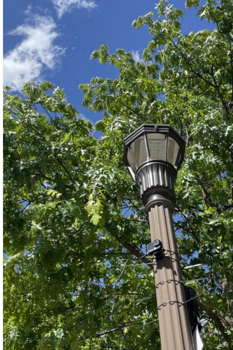
Figure 2. Video Camera Installed on a Campus Street Light
