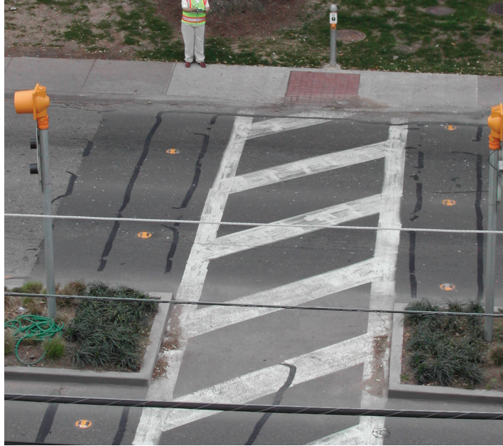
Figure 10-11. Photo. Working example of in-roadway warning lights with pedestrian pushbutton in Austin, TX.
