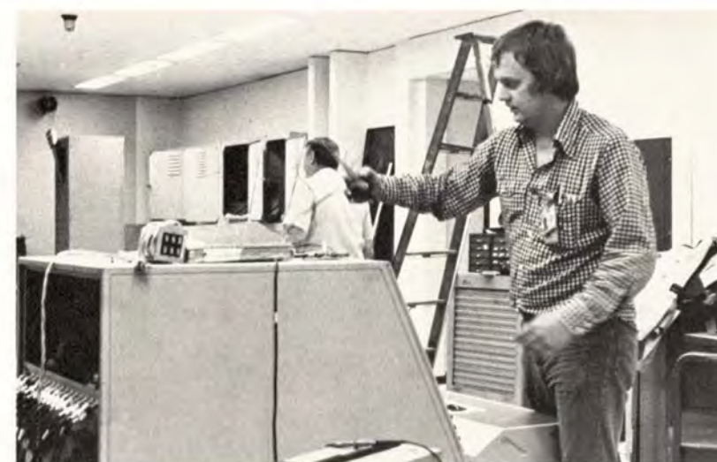
Installation specialist Mike Bezdov adjusts a vertical radar display in the simulation lab. Resident engineer Ed Hock is in the rear.
