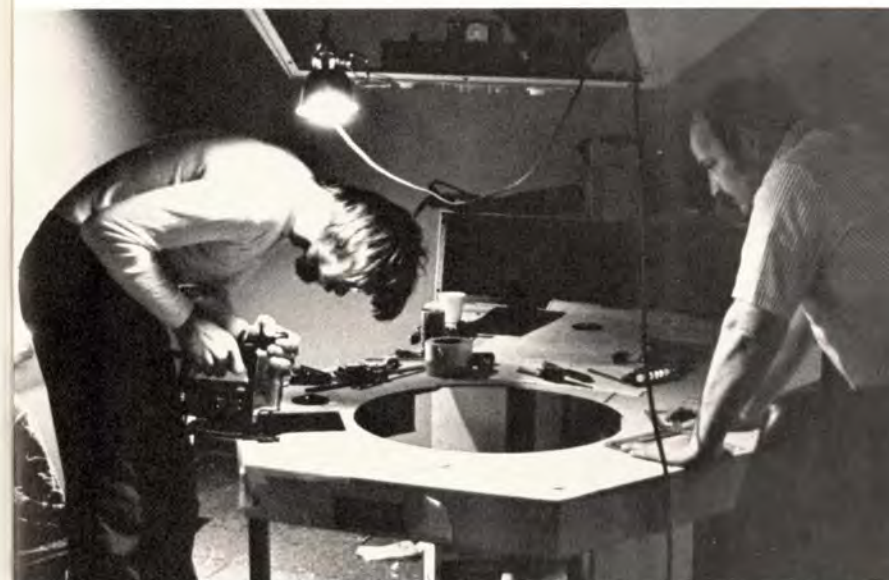
Airway Facilities technicians Steve Diedrich (left) and Tom Couch are among the specialists who designed and installed the equipment in O'Hare Airport's simulation laboratory.
