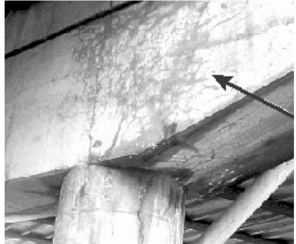
The gradual formation of the mineral ettringite has been associated with cracking in concrete, such as the damage shown here.
