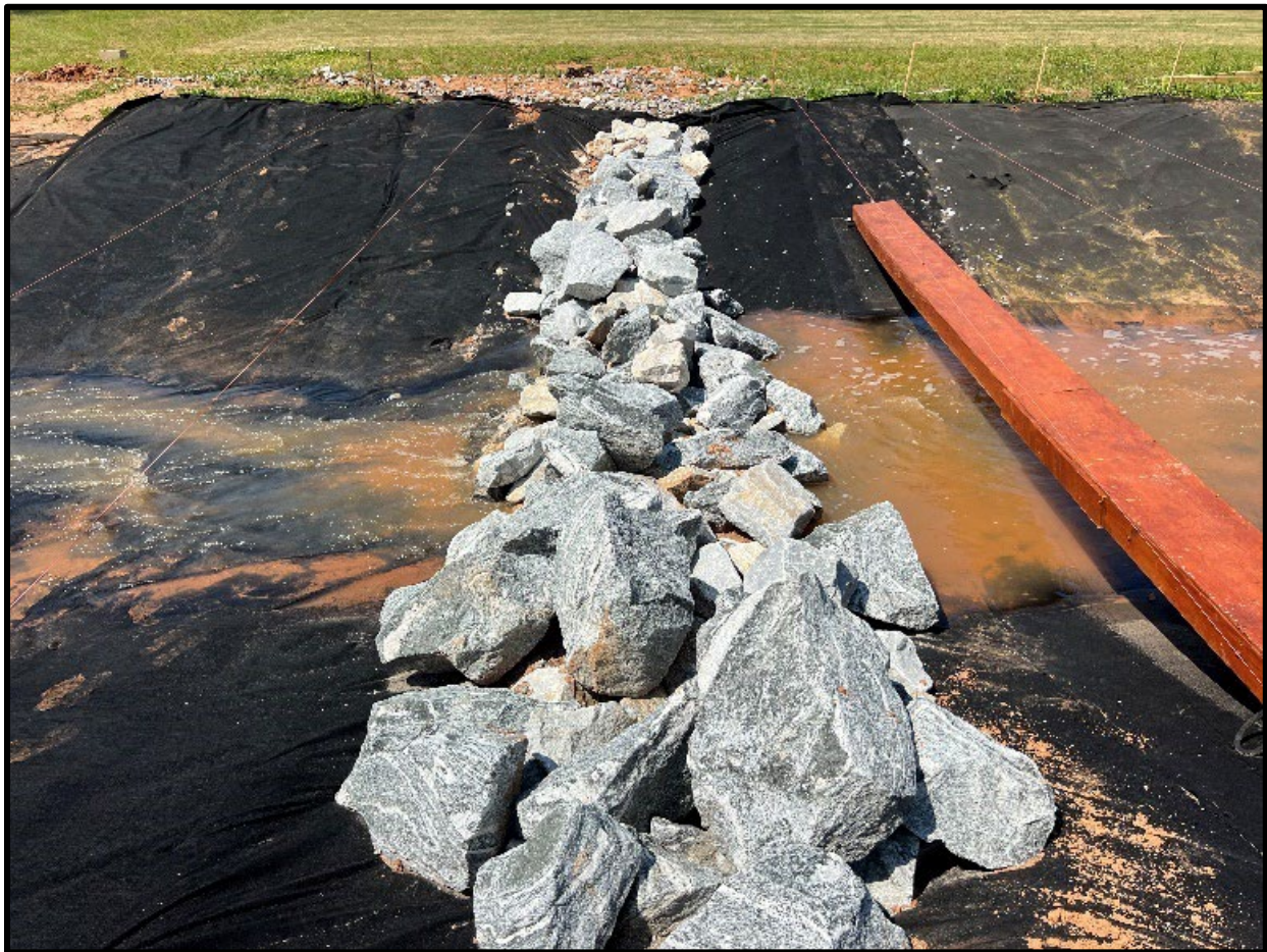
Figure 4.1: Upstream Impoundment of Iowa DOT Standard Installation
