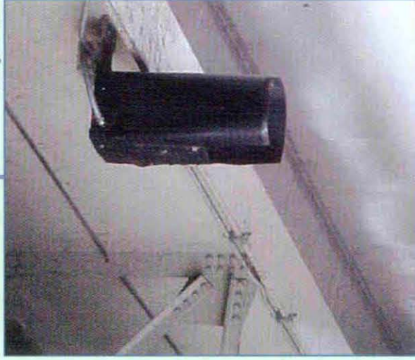
Fully shielded light fixture on the I-405 Bridge
