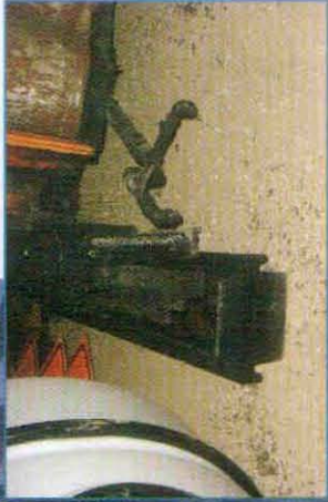
Basin catches drips or spills from equipment
