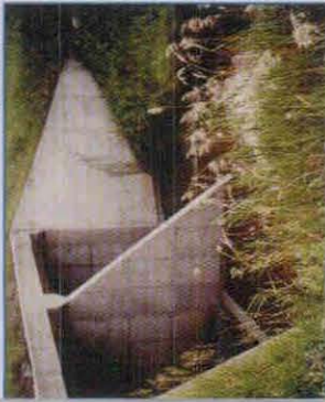
Double box culvert with “lip” to divert low flows into single barrel
