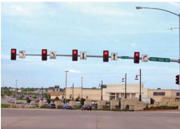
Figure 3: Example Intersection with Basic 12 inch Lens, Back Plates and a Signal Head per Lane
