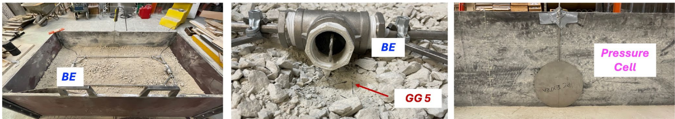
Figure 50. Photo. BE field sensors and pressure cell placement.
