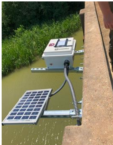
Figure 73. BIN 007070, Demopolis, AL. Enclosure and Solar panel.
