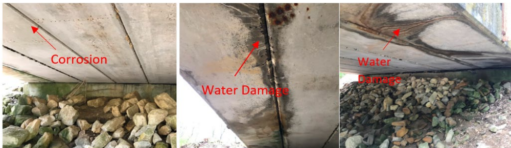
C. Corrosion and water damage under the deck
