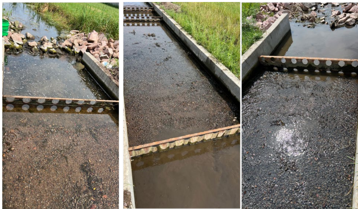
Figure 3.17 Filter structure after filter maintenance
