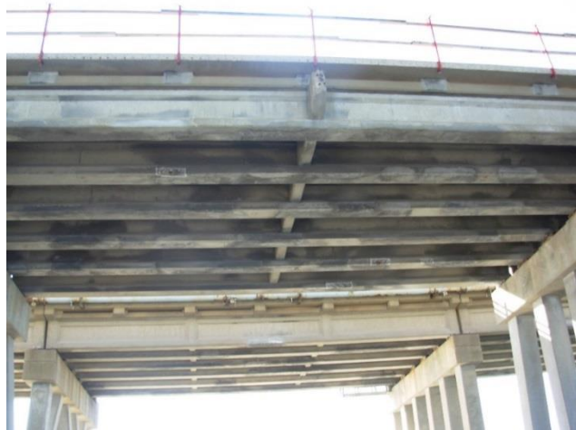
Figure 1. Typical Deterioration on the Lesner Bridge
