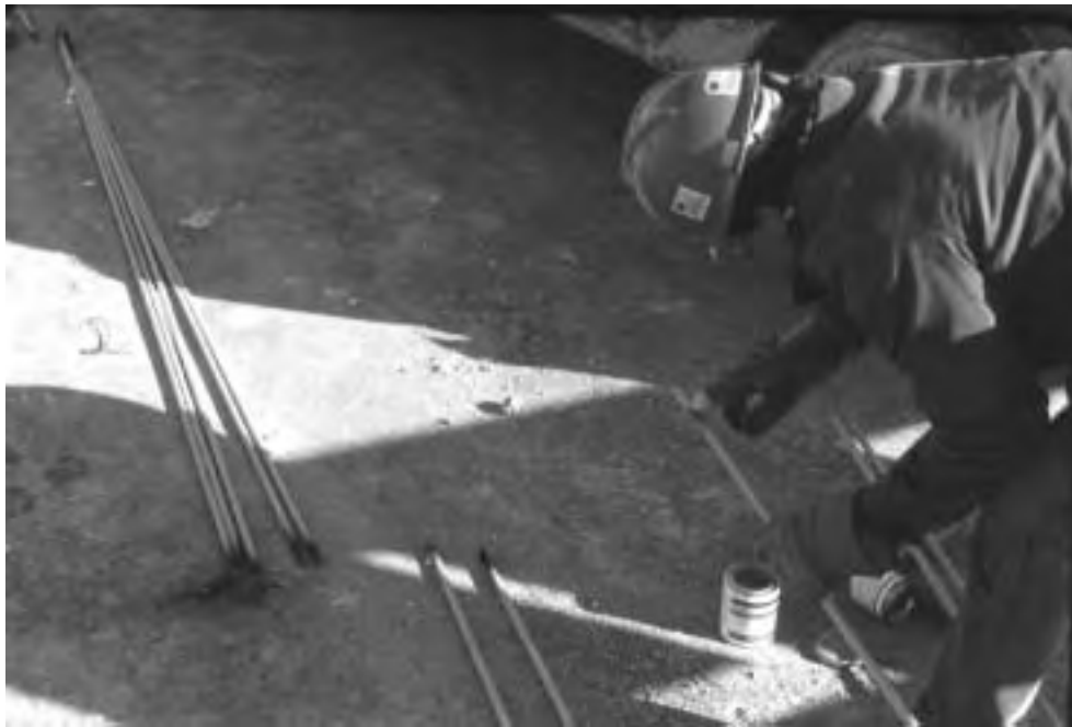
Figure 1.6 Improper field practice: Epoxy coated bars were flame cut and, immediately thereafter, bar ends are being touched up by hand.
