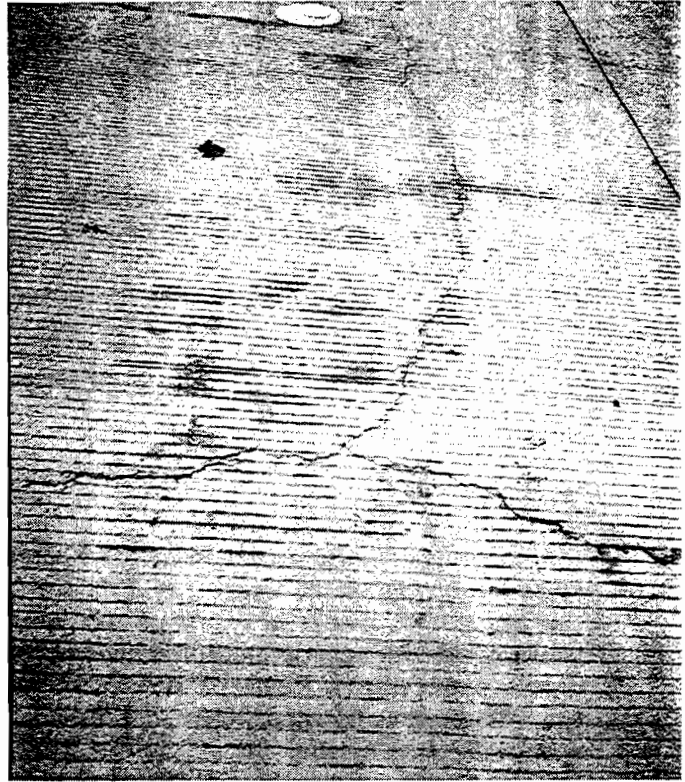
Figure 4.9 Typical longitudinal crack occurring with summer placements (SH 6 summer)
