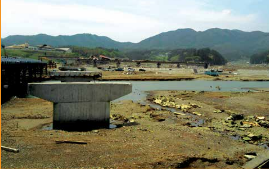
(Left) Shown here are bridge superstructures (girders and decks) washed out by the tsunami generated by the Tohoku Earthquake in Japan in 2011.
