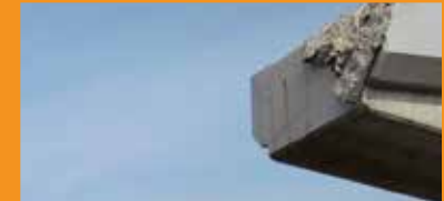
(Below) This bridge located along Japan's northeast shore was severely damaged, including superstructures washed out and piers displaced by the tsunami wave from the 2011 earthquake.
