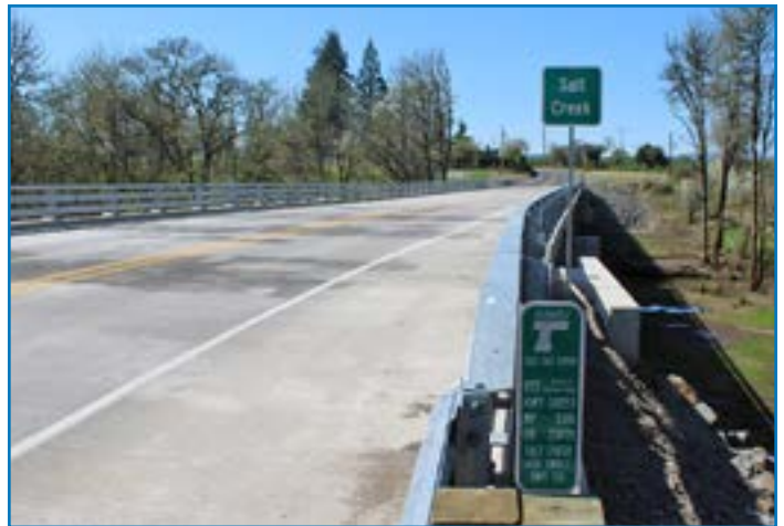
The Salt Creek Bridge was one of several internally cured bridge deck projects the Oregon DOT surveyed that showed significantly less shrinkage cracking versus traditionally cured concrete decks.
