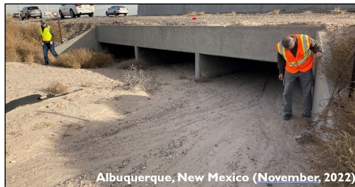
Figure 14. Sedimentation conditions at three-box culverts: a) IMM group; b) NMU group
