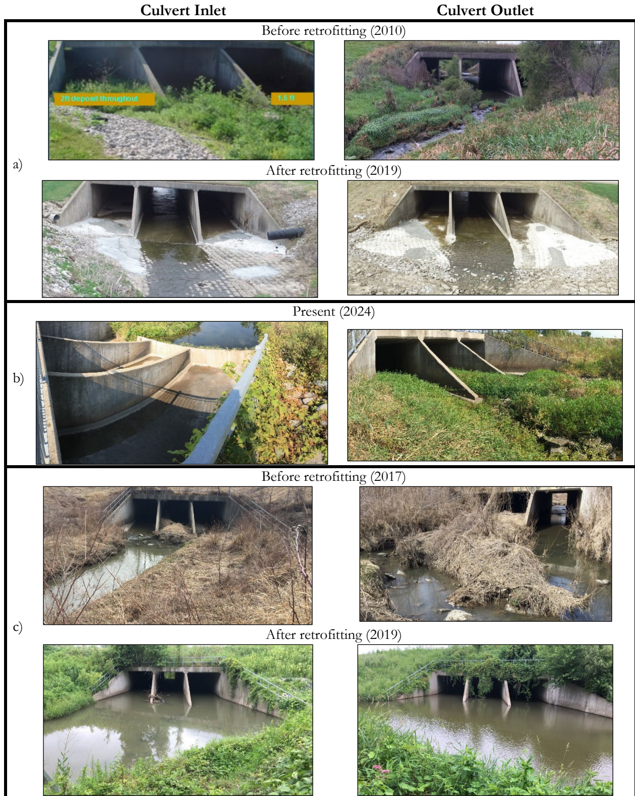
Figure 9. Self-cleaning culvert solutions: a) Design A (fillet-based) applied to a triple 15'-18'-15x12' ~ 170-ft long culvert; b) Design B (upstream downward curtain) applied to a triple 15'-18'-15x12' ~ 800-ft long culvert; c) Design C (downstream weir) used for a Triple 15'-18'-15x12', ~ 200-ft long culvert
