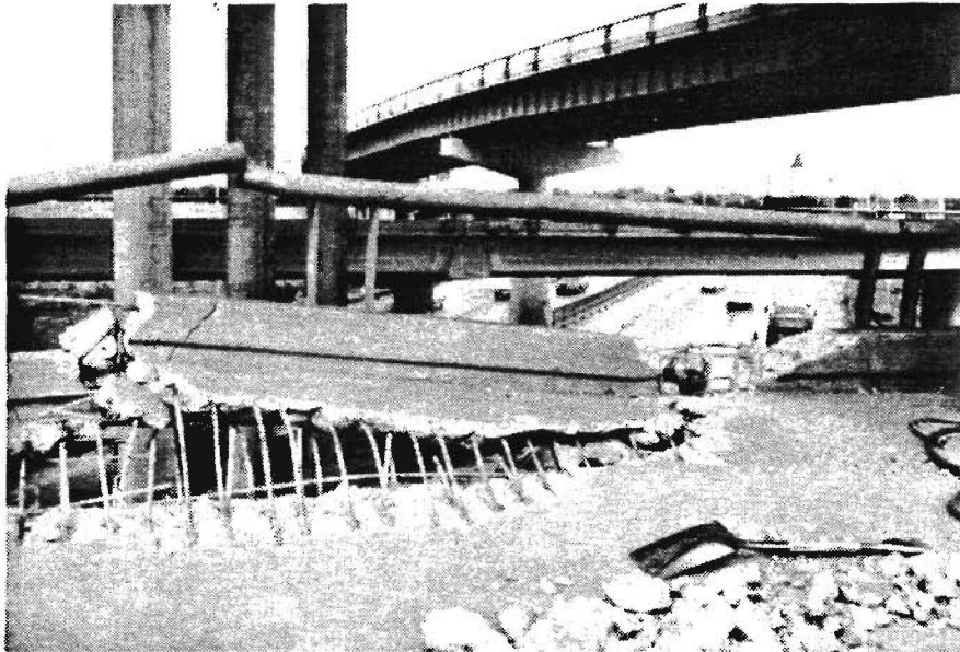
FIG. 1. Damaged Bridge Slab and Safety Rail
