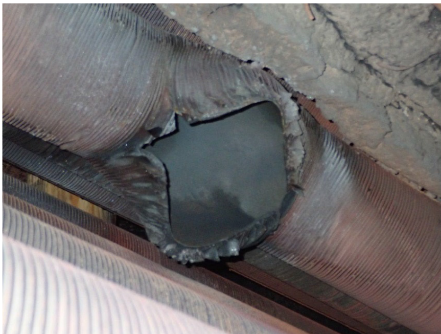
Figure 7. Ruptured fired heater tubing. (Credit: Valero)
