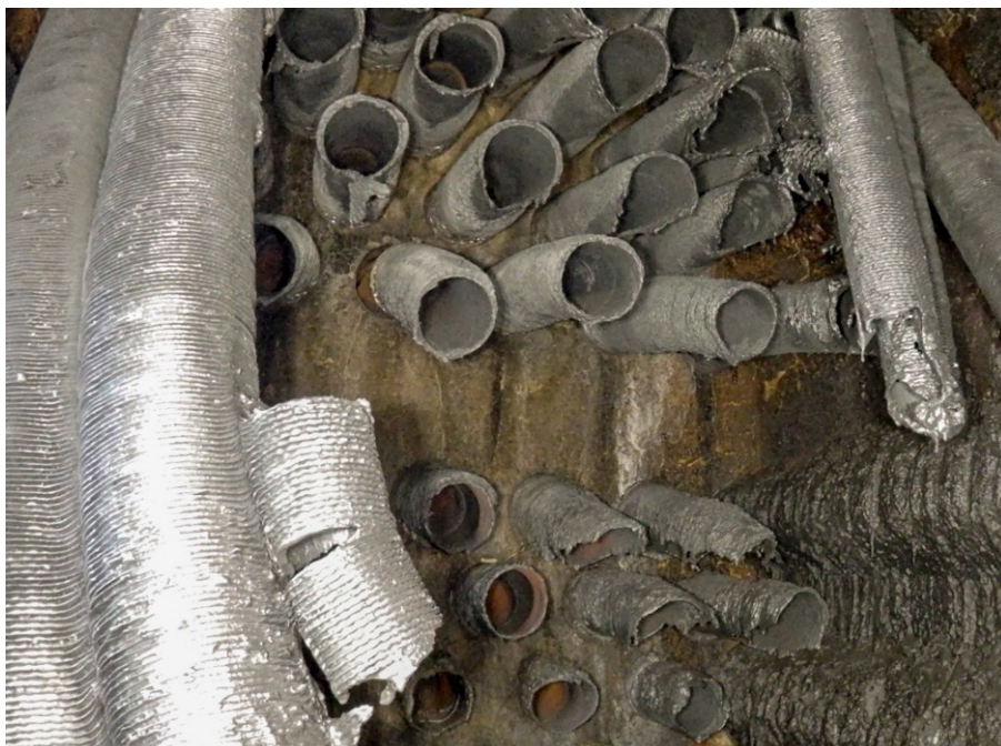
Figure 19. Broken fired heater tubes. (Credit: LyondellBasell)
