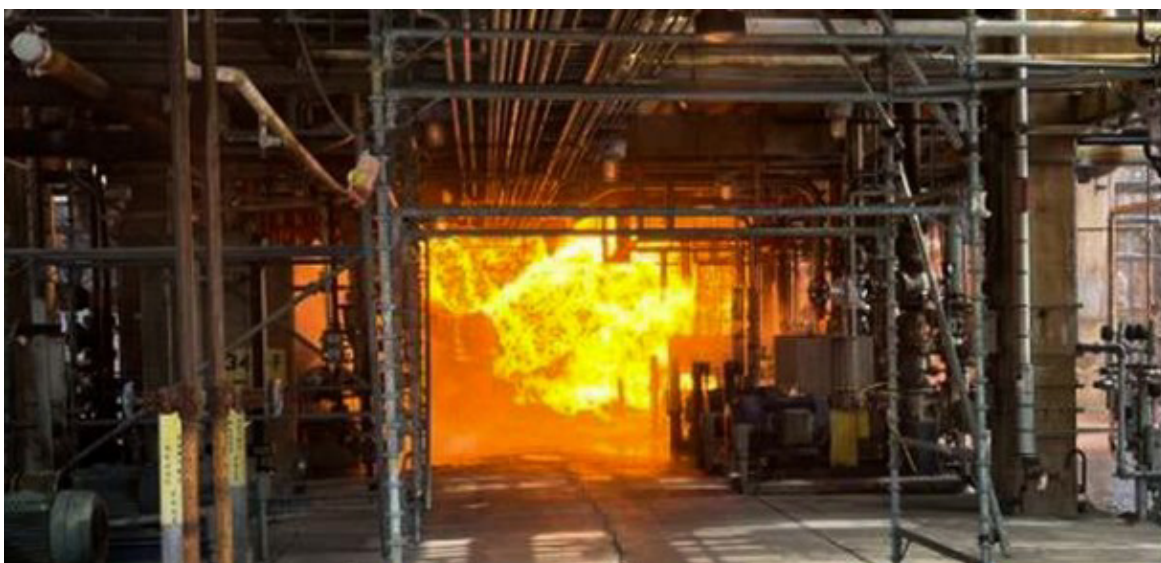
Figure 14. Fire from breached piping. (Credit: Marathon)
