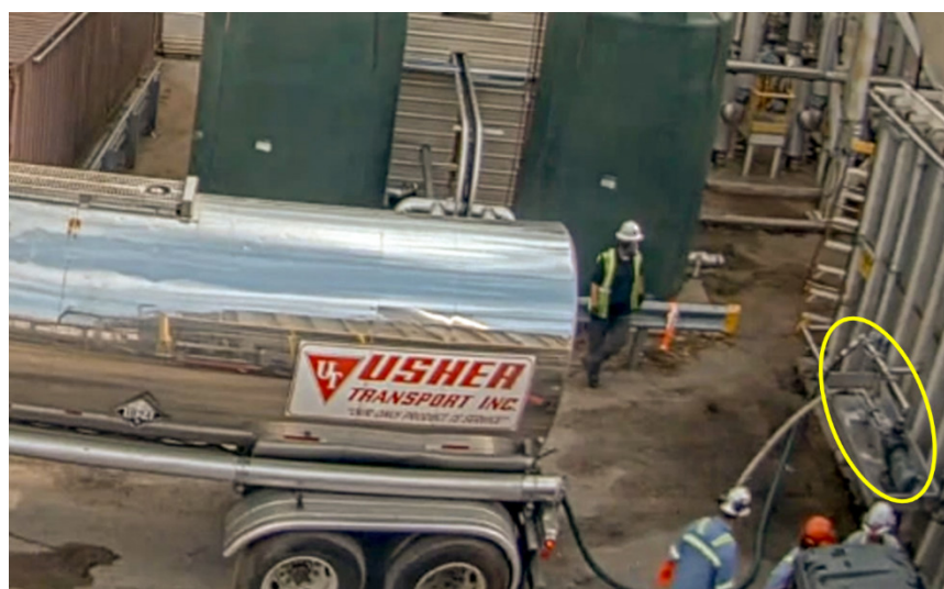
Figure 1. Caustic Unloading Pump (yellow oval). (Credit: Georgia-Pacific)
