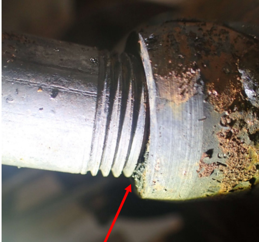
Figure 2. Damaged Mineral Oil Piping. (Credit: Chemtool)
