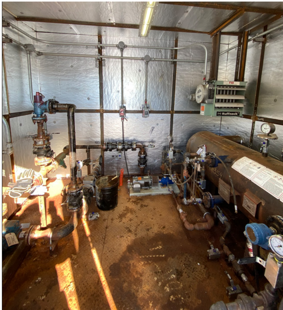
Figure 1. The Enclosed Building. (Credit: ConocoPhillips)
