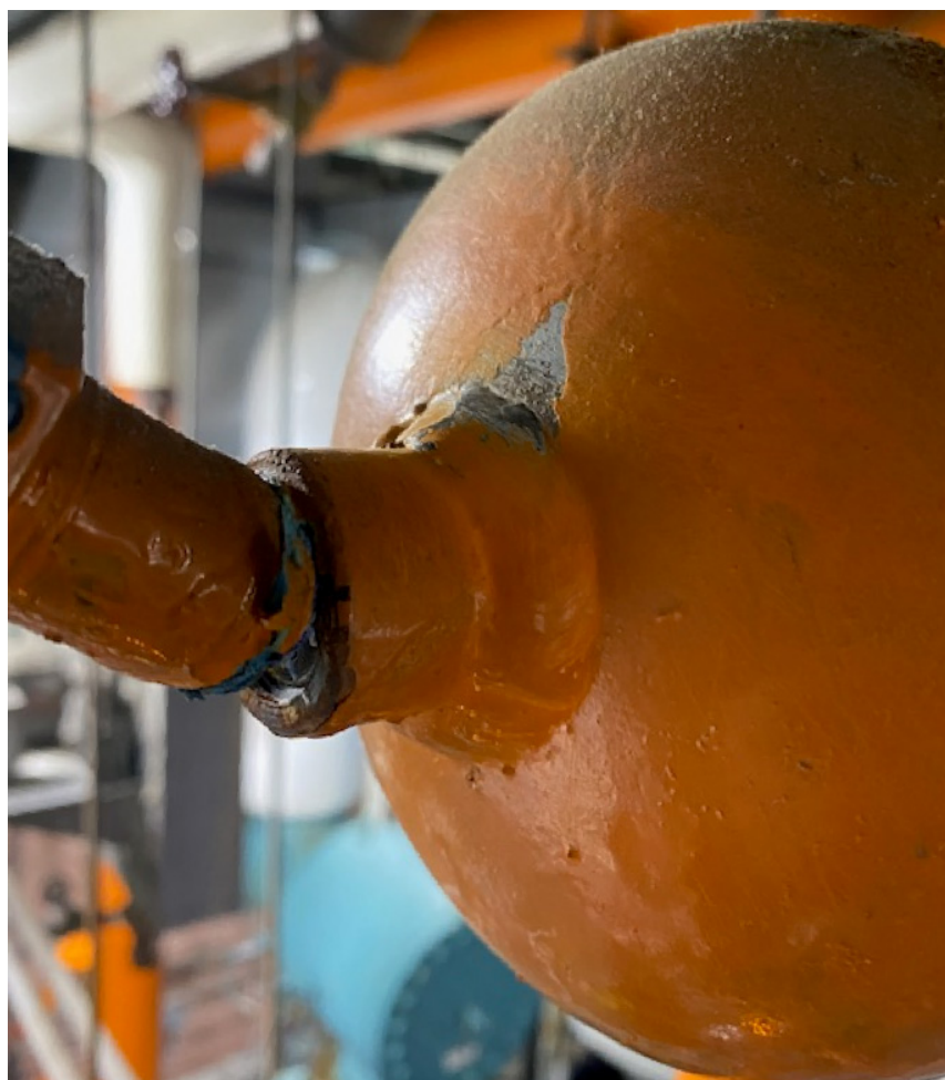
Figure 1. Damaged Ammonia Piping. (Credit: HMF)
