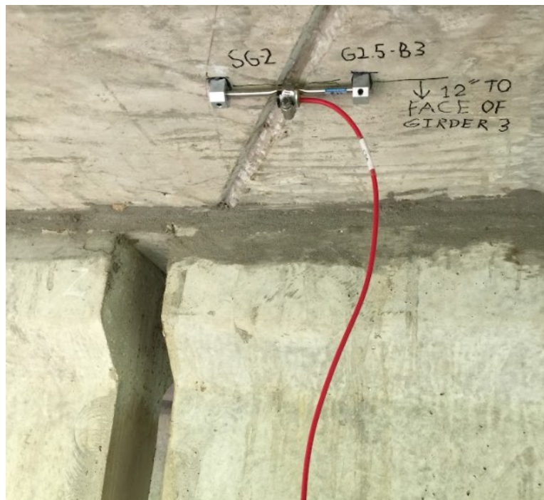
Figure 6.10. A poor boy continuous deck above girder ends on a skewed support at Old River Bridge, without the use of foam insert or skewed end girder detail.
