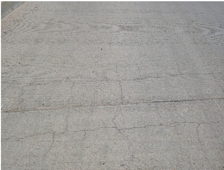
(c) Marked cracks in NDE area
