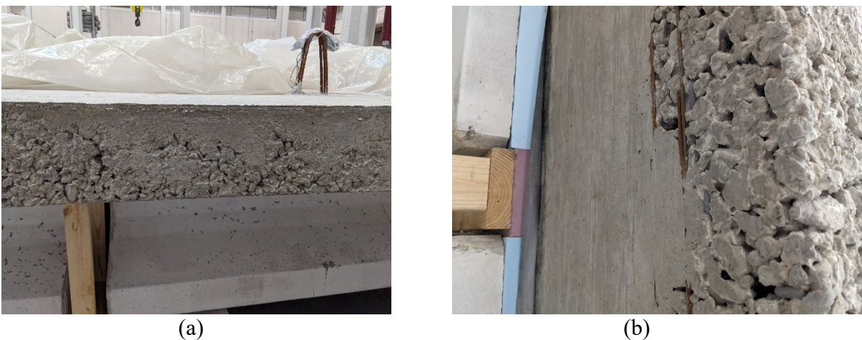
Figure 9.34. PBJ-CP1 honeycombing in south overhang prior to repair.
