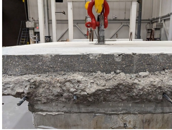
Figure 9.55. PBJ-OP1R: Post-test demolition view of concrete over east girder showing horizontal crack at mid-depth.
