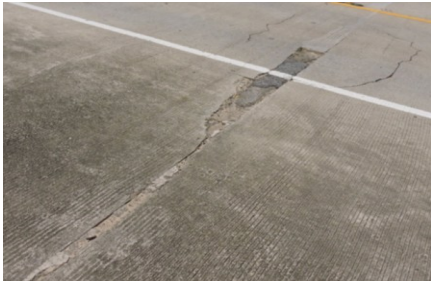
(a) Cracking and spalling on top of deck
