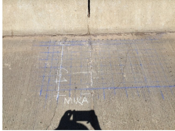
(b) Marked cracks in overhang
