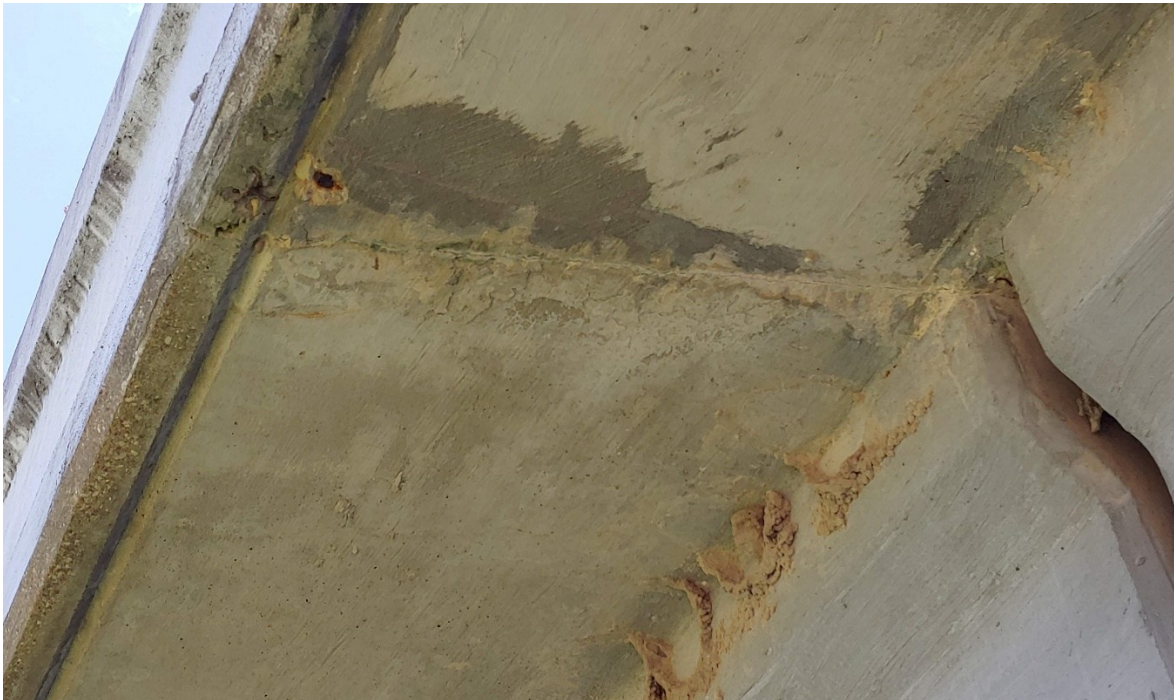
Figure 6.12. Cracking in the deck above the girder ends at skewed supports on Peach Creek Bridge.
