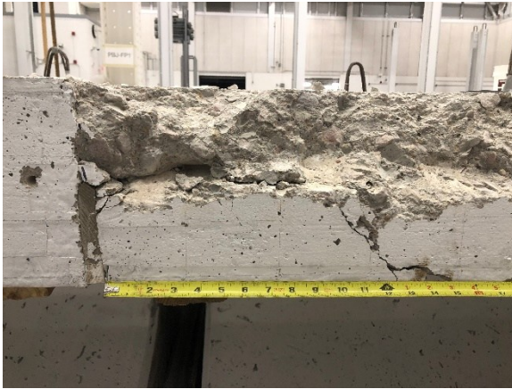
(a) Crack in southeast overhang
