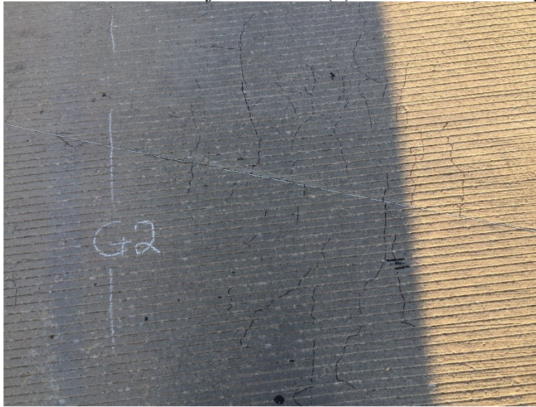
(c) Marked cracks in NDE region
