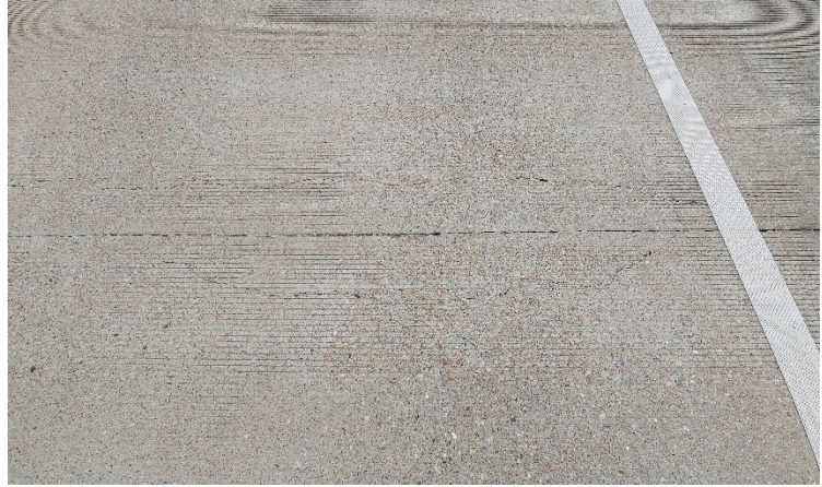
(b) Main and secondary PBJ cracks
