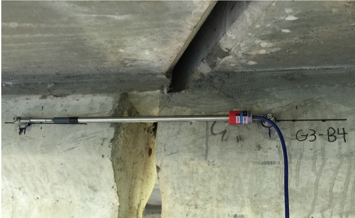
Figure 6.11. Contact between girder end and the deck of the adjacent span at an expansion joint on Old River Bridge.
