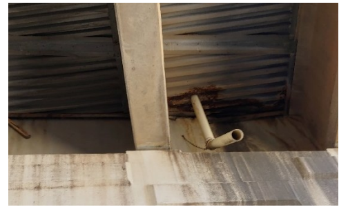
(b) Rusting PMDF on eastbound side
