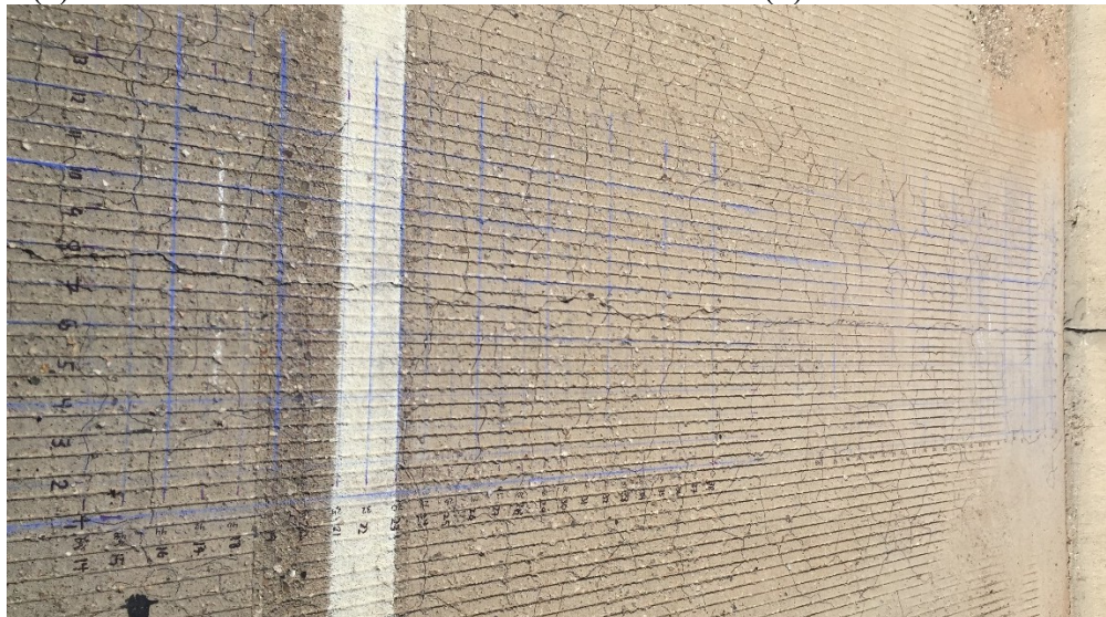
(e) Marked cracks in NDE regions
