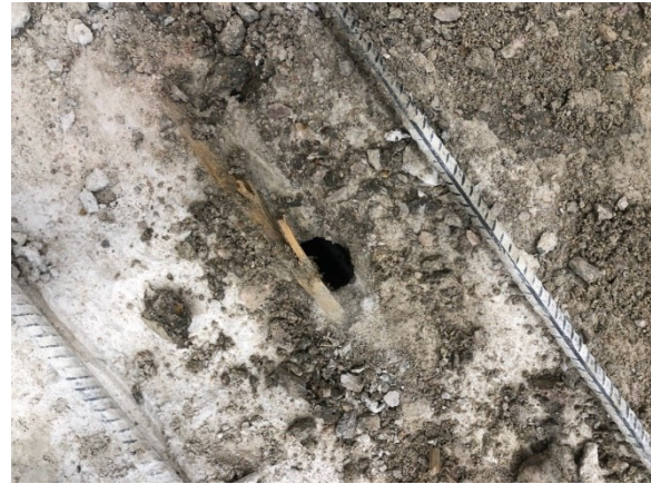
(b) Hole adjacent to board between north girders
