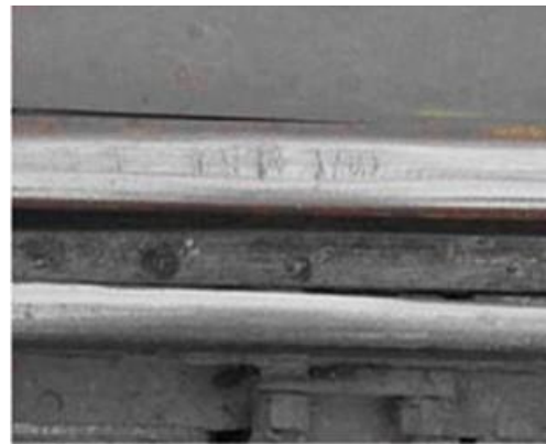
Thermal cracks on burned stock railhead
