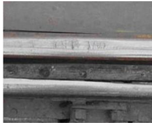
Thermal cracks on burned stock railhead
