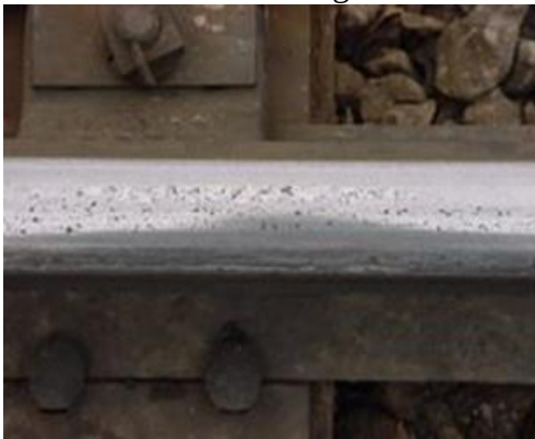
Flaking caused by centralized loading
