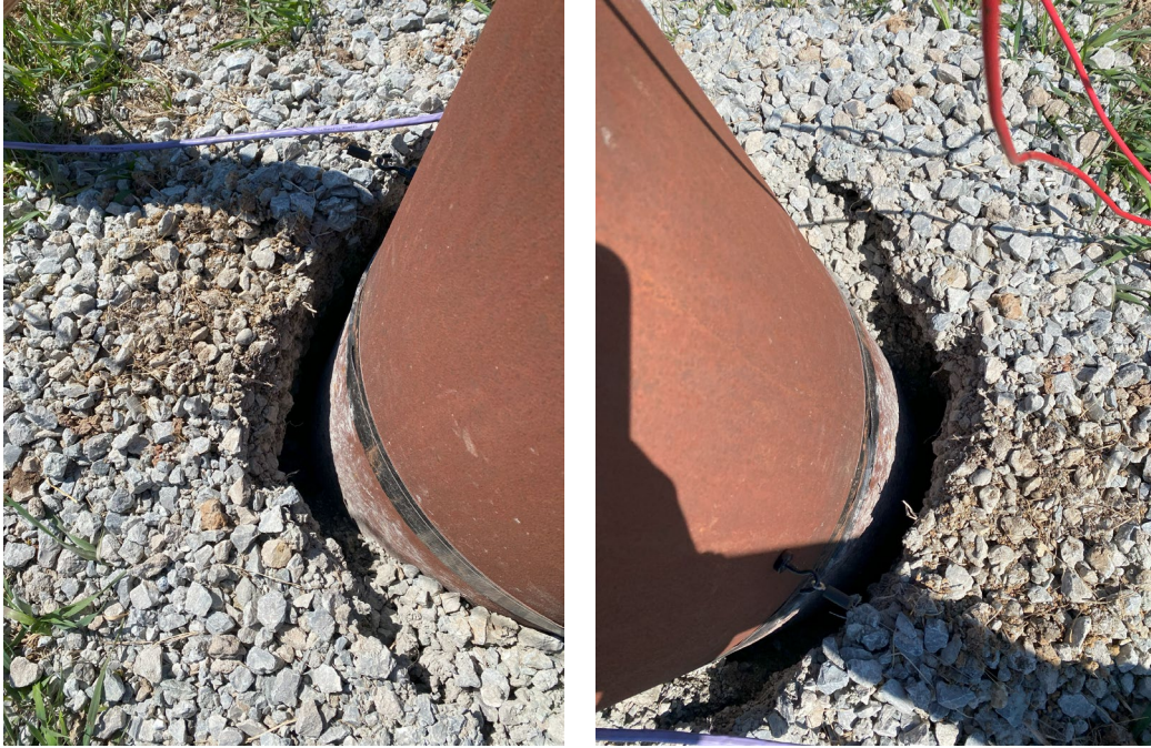
Figure 6.33 Observed damage in poles with gravel backfill after static tests
