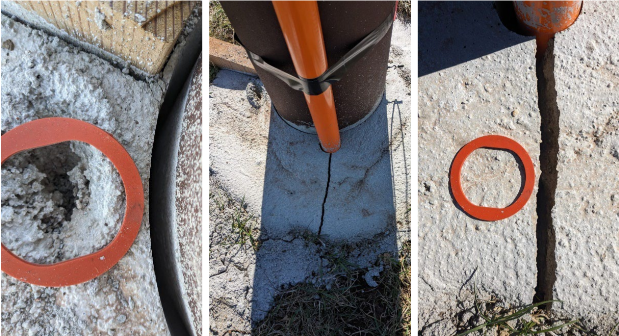
Figure 6.32 Observed damage in poles with concrete backfill after static tests
