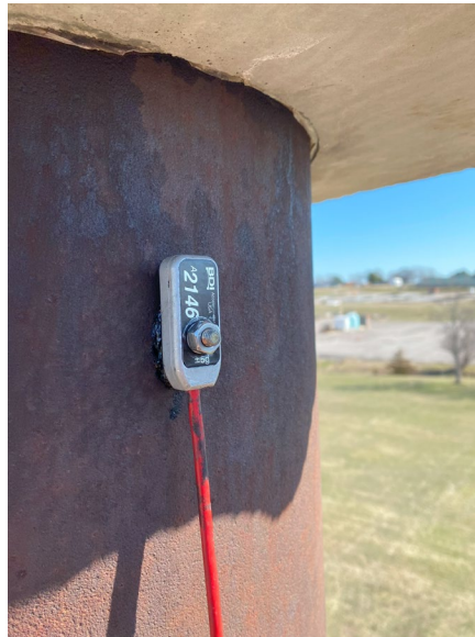
Figure 4.11 Accelerometers used to measure the acceleration at different locations during dynamic tests
