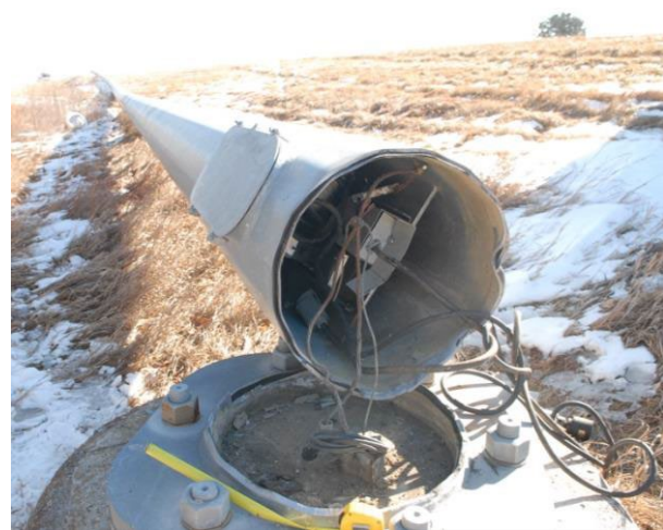
(b) High-mast Tower Failure (cite)
