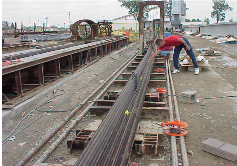
Figure 3. Magnetoelastic sensors installed on a strand
