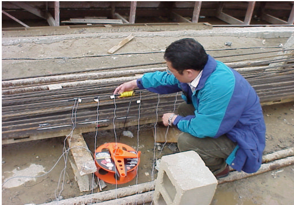
Figure 4. Magnetic sensor (colored in yellow) installed on a strand
