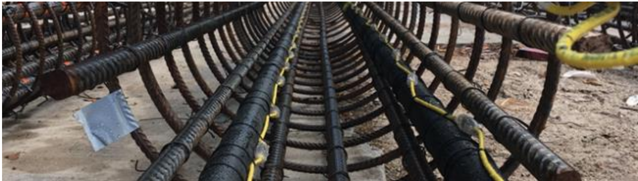
Figure 1.10 Thermal wires (yellow) tied along the length of an auger cast reinforcement cage
