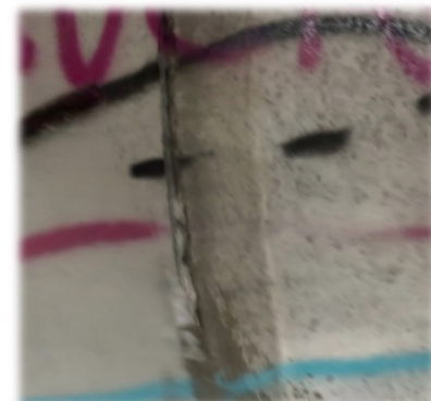
Figure 6. Screenshot. Closeup of spalling at a joint in the culvert in the texture-mapped mesh.
