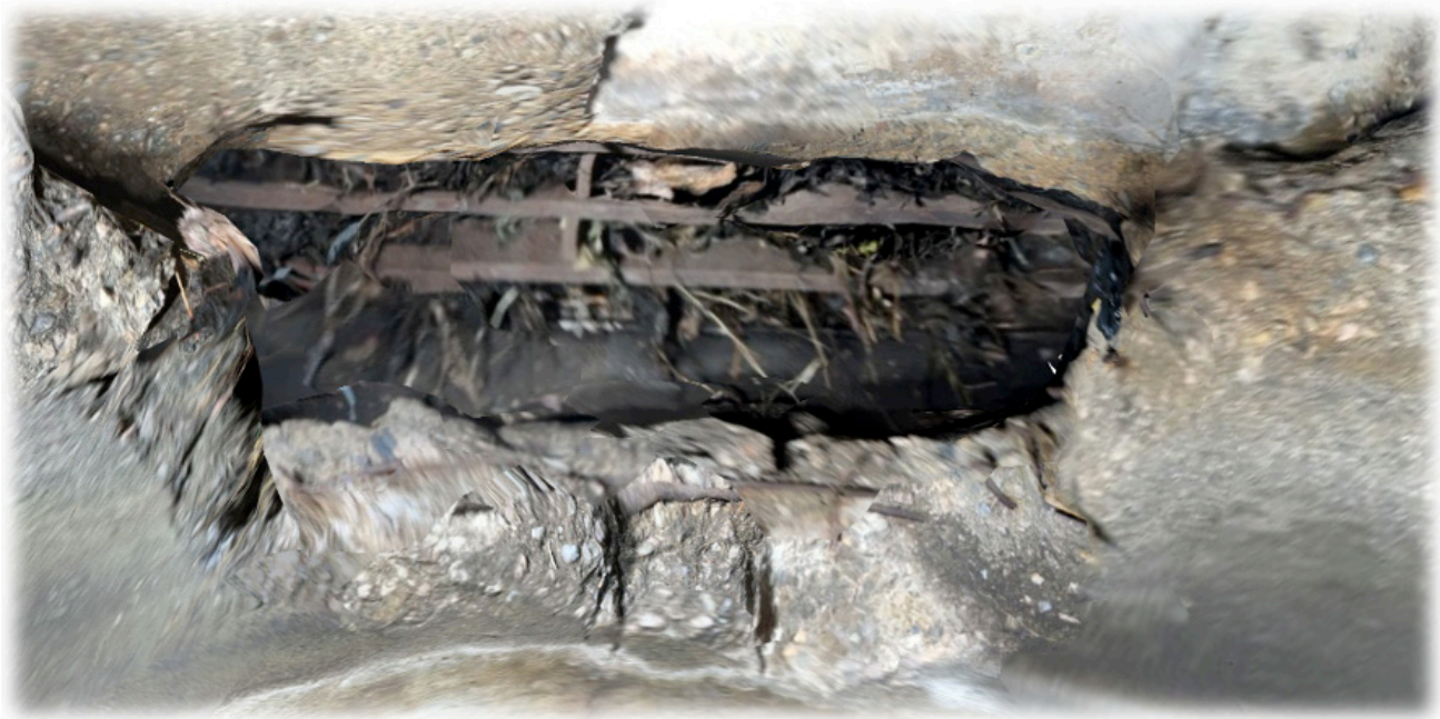
A. Clogged catch basin near the inlet.
