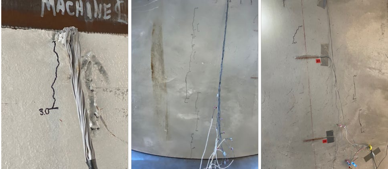
Figure B4-8: Damage of segment after test 4 completion.
