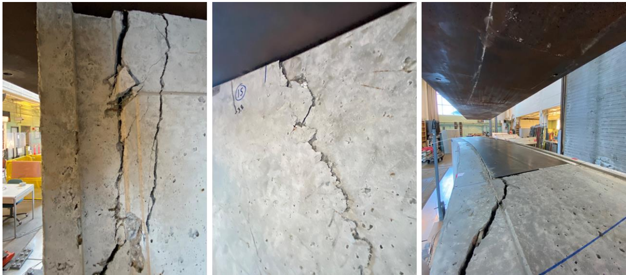
Figure B3-7: Damage of segment after test 3 completion.
