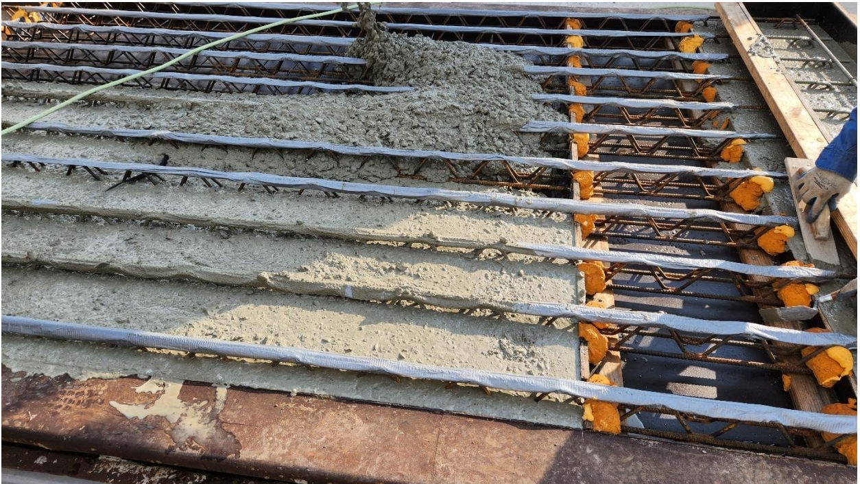
Figure 6-1: Duct tape covering top chord rebar
