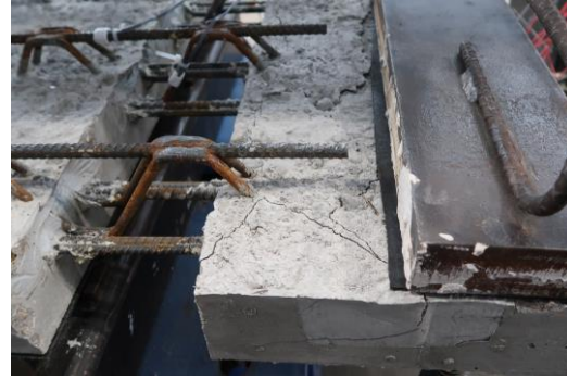
(b) After flexural and shear cracks develop in concrete during load testing
