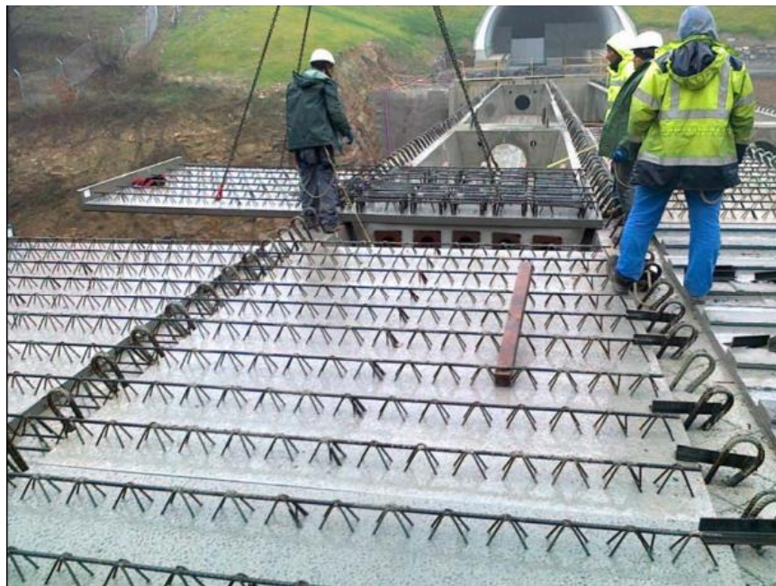
Figure 2-9 Lattice girders continuous over the fascia girder (a)courtesy of Roads and Bridges LLC, (b) courtesy of Dr. David Fernández-Ordóñez
