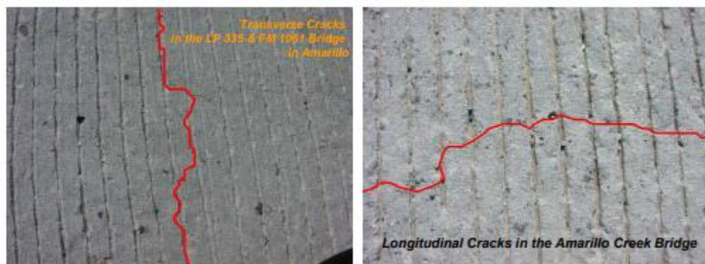
Figure 2-2 Typical deck cracking observed by Shoemaker et al. (2002)
