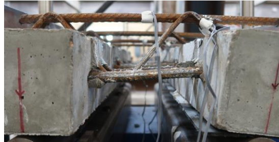
(b) Wire trusses slip out of the panels during loading
