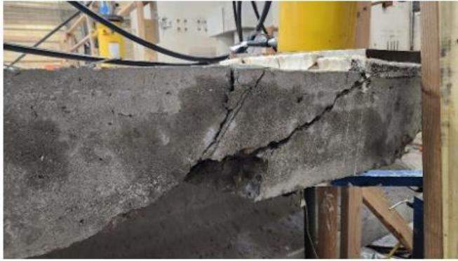
(a) Shear crack from free edge
