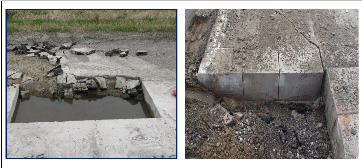
Figure 1.1 PCC on non-drainable MnDOT Class 5 gradation base (left) vs Permeable Asphalt Stabilized Base (a drainable base) (right).
