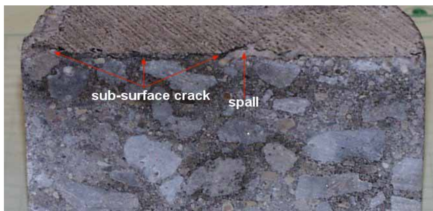
Figure 15. Development of spall as a result of early application of curing compound.
