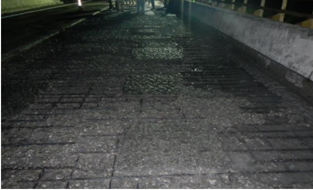
(a) Bridge deck after hydro-blasting and vacuuming showing patched concrete remaining above the upper mat of reinforcing steel
