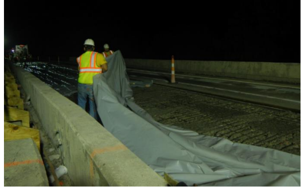
(b) Workers placing plastic sheets on prepared deck to prevent contamination of the prepared surface prior to overlay placement
