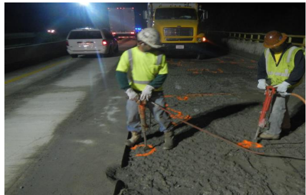
(f) Jackhammering to remove unsound or delaminated concrete detected by the chain drag method after hydro-blasting; resulting debris collected by vacuum truck
