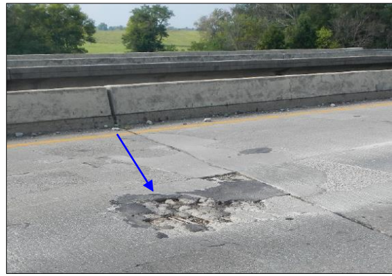
(b) Deck surface showing exposed reinforcement steel (marked with an arrow)
