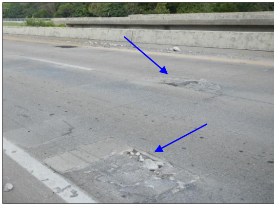
(a) Portion of a deck surface showing spalling on the riding surface (marked with arrows)
