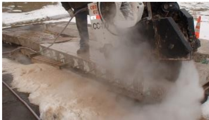
Figure 4. Cutting the first Concrete Panel to allow for cross sectional view of grout distribution
