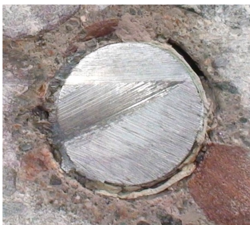
Figure 17. Dowel Hole Location 5 - Significant Reflection with Some Voids Present
