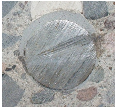
Figure 19. Dowel Hole Location 22 - Little to No Reflection with No Voids Present
