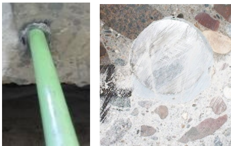
Adhesive Sample Test Hole #17 - Epoxy filled hole and applied bead of epoxy to dowel
