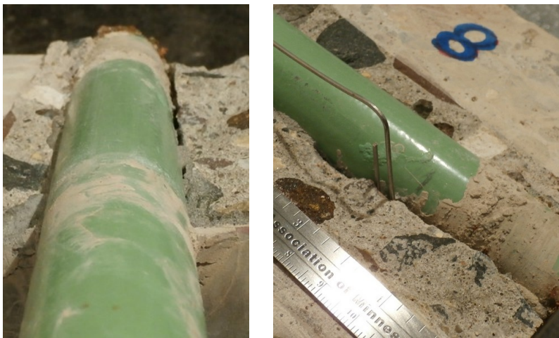
Adhesive Sample Test Hole #8 - Non-Shrink Grout, used past recommended application time
