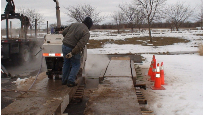
Figure 6. Making the final forensic cut on the first concrete panel (both sides of the second panel had been completed)
