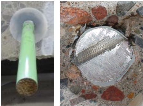
Adhesive Sample Test Hole #14 - Epoxy filled hole and applied bead of epoxy to dowel
