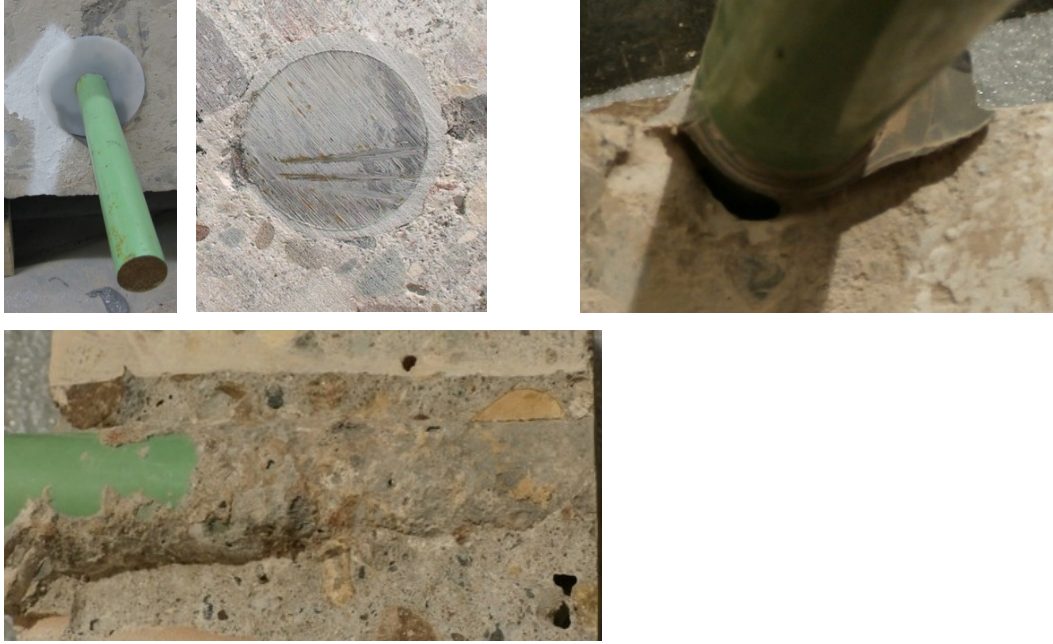
Adhesive Sample Test Hole #24 - Poly-Grip is a two-component epoxy – 20 'Pumps' of adhesive
