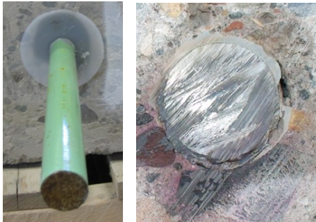
Adhesive Sample Test Hole #12 - Epoxy filled hole and applied bead of epoxy to dowel
