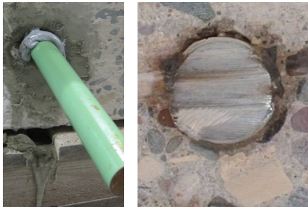
Adhesive Sample Test Hole #40 – Non-Shrink Grout in combination with Single Dip Two Part Epoxy, Hand Mixed
