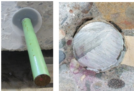
Adhesive Sample Test Hole #18 - Epoxy filled hole and applied bead of epoxy to dowel
