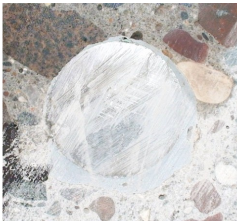
Figure 16. Dowel Hole Location 17 - Slight Reflection with No Voids Present
