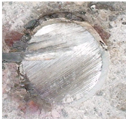
Figure 15. Dowel Hole Location 6 - Significant Reflection with Little to No Voids Present
