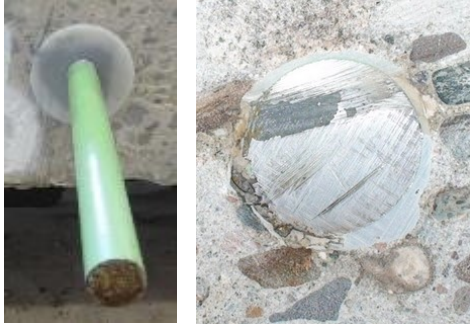
Adhesive Sample Test Hole #16 - Epoxy filled hole and applied bead of epoxy to dowel
