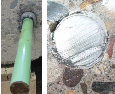
Adhesive Sample Test Hole #13 - Epoxy filled hole and applied bead of epoxy to dowel
