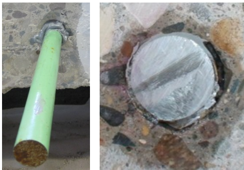
Adhesive Sample Test Hole #15 - Epoxy filled hole and applied bead of epoxy to dowel
