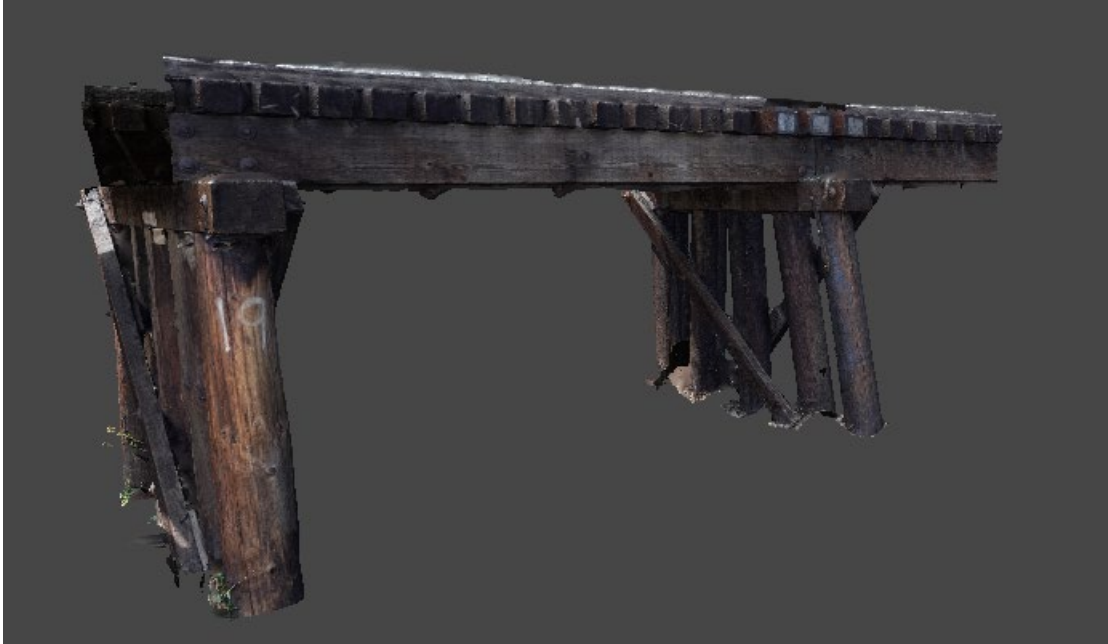
Figure 2.8 Final SfM image of railroad bridge in northern Fort Collins. This is a two-dimensional capture of the full three-dimensional model that can be viewed from any angle or orientation/height.
