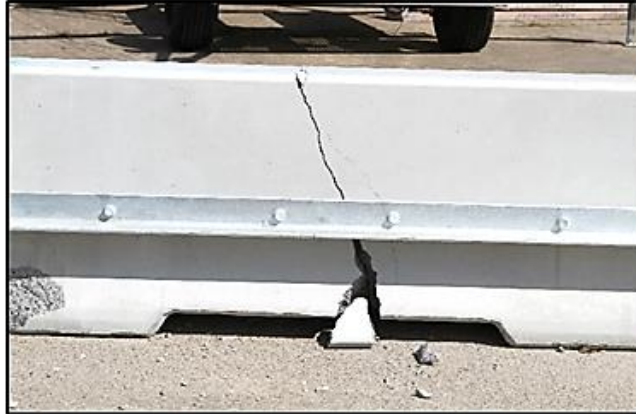
Figure 2.15. Concrete Crack after MASH Test 3-11 on MassDOT Retrofit PCB System (27).
