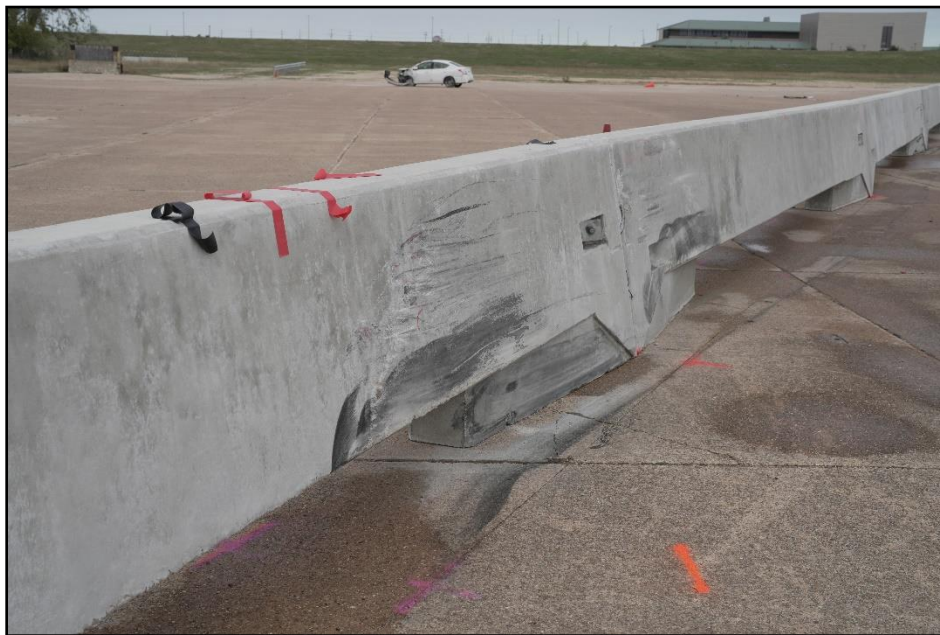
Figure 9.5. Large-Scupper Portable Concrete Barrier after Test at Impact Location for Test 440873-01-1.
