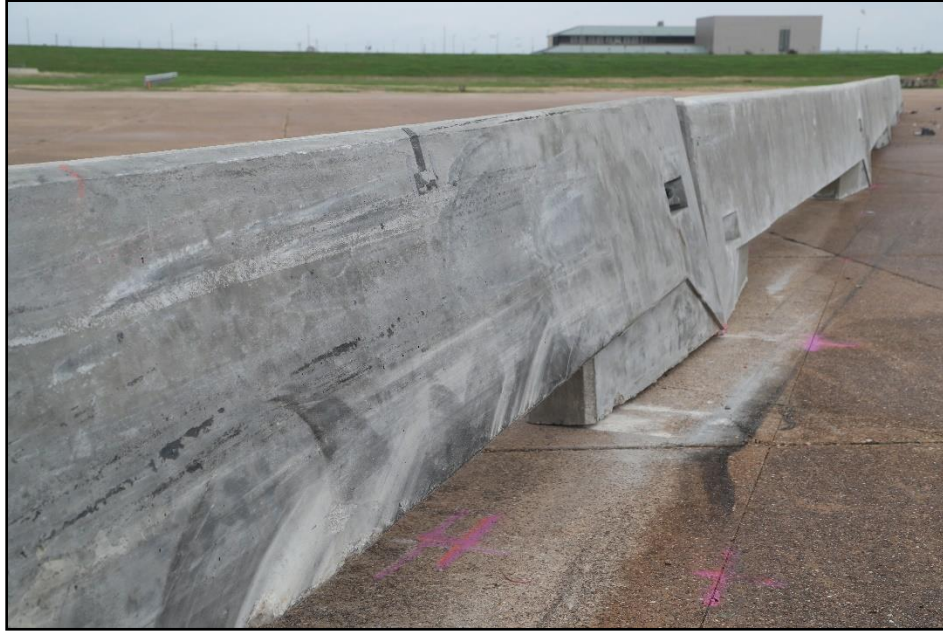
Figure 10.6. Large-Scupper Portable Concrete Barrier at the Joint of Barriers 3 and 4 after Test 440873-01-2.
