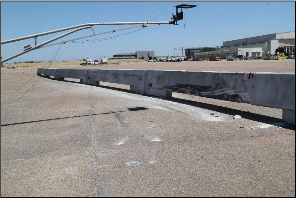
Figure 11.5. Large-Scupper Portable Concrete Barrier at Impact Location after Test 440873-01-3.
