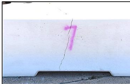
Figure 2.14. Concrete Crack after MASH Test 2-11 (27).
