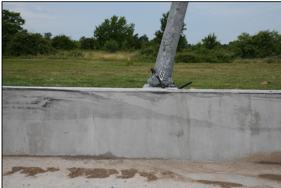
Figure 5.6. Traffic Side View of the Damage to the Base of the Luminaire Pole after Test 440863-03-1.
