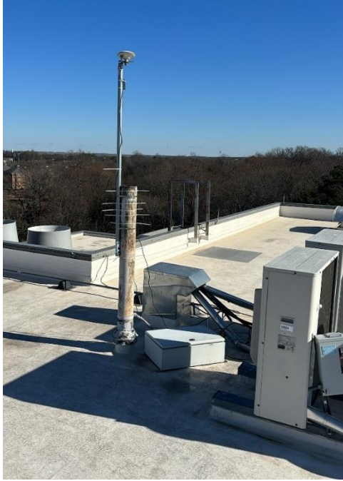
Figure 3. GNSS antenna installed on the roof of McEniry Hall on UNC Charlotte's main campus. (Image courtesy of Beep)
