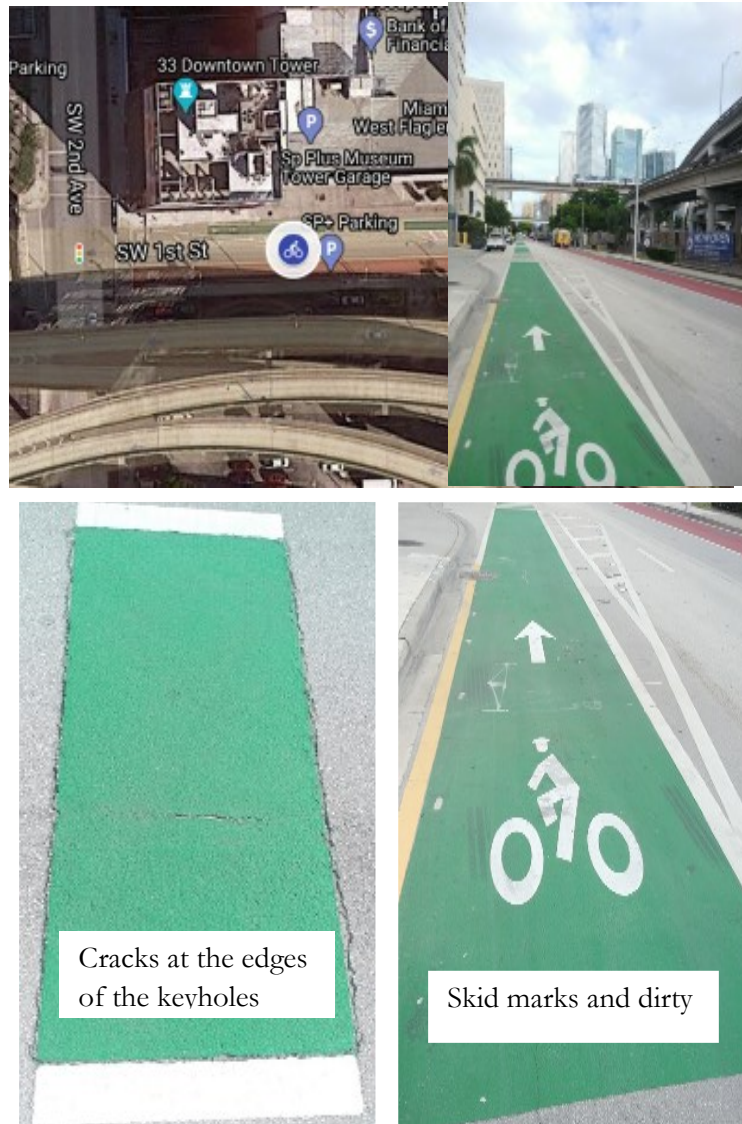
Figure A-23. Site 59-Location and Distresses.
