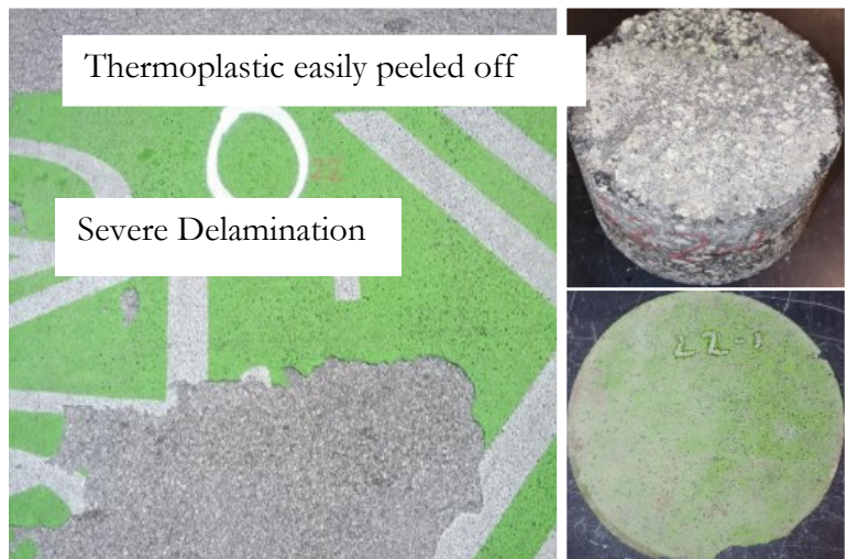
Figure A-5. Site 22-Location and Distresses.
