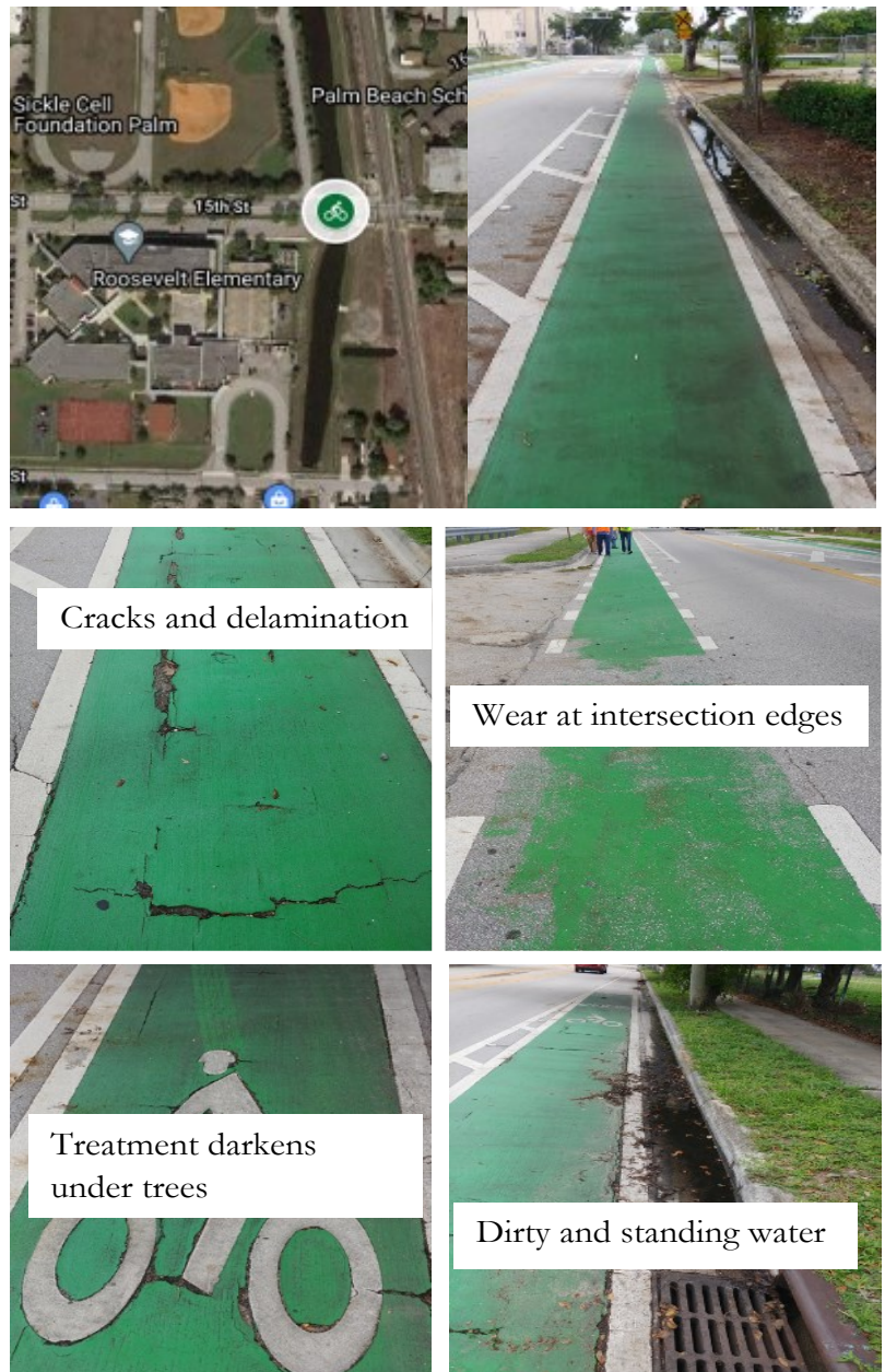
Figure A-15. Site 17-Location and Distresses.
