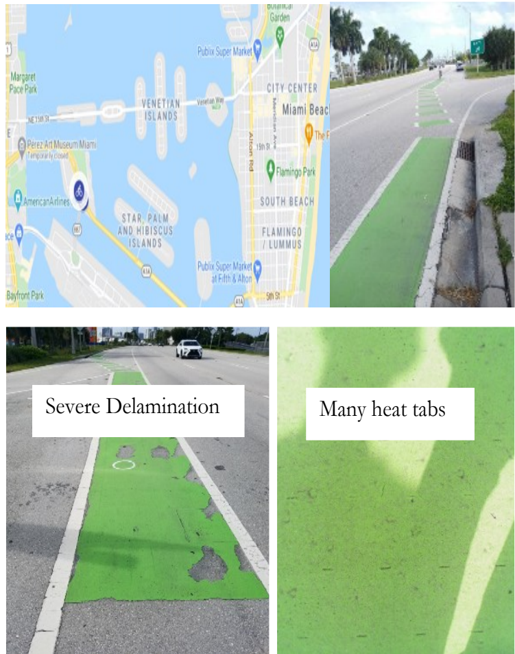
Figure A-7. Site 28 and 29-Location and Distresses.
