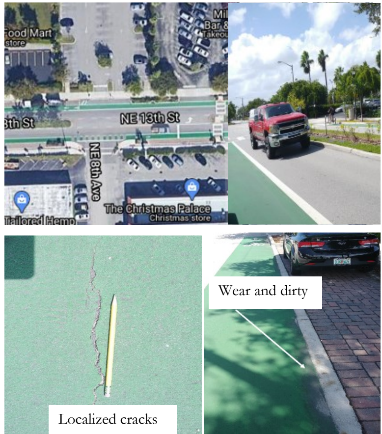
Figure A-22. Site 56-Location and Distresses.
