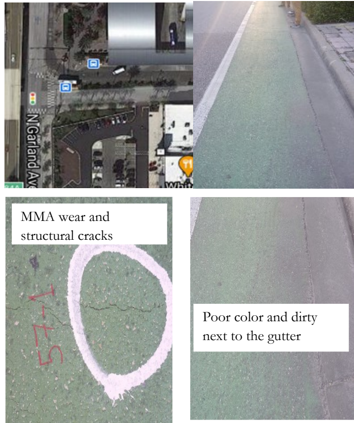
Figure A-27. Site 57-Location and Distresses.
