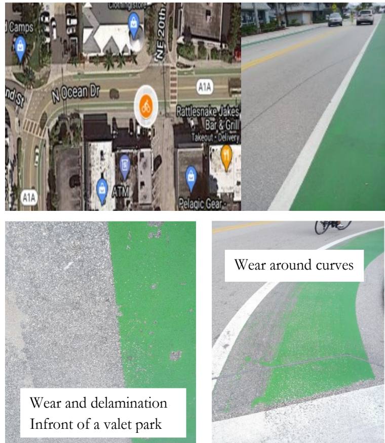
Figure A 20. Site 21-Location and Distresses
