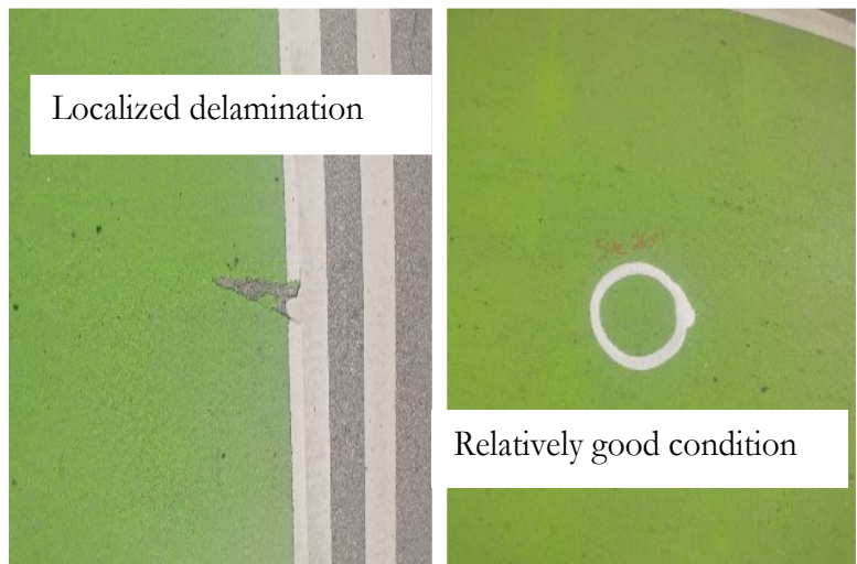
Figure A-4. Site 26-Location and Distresses.
