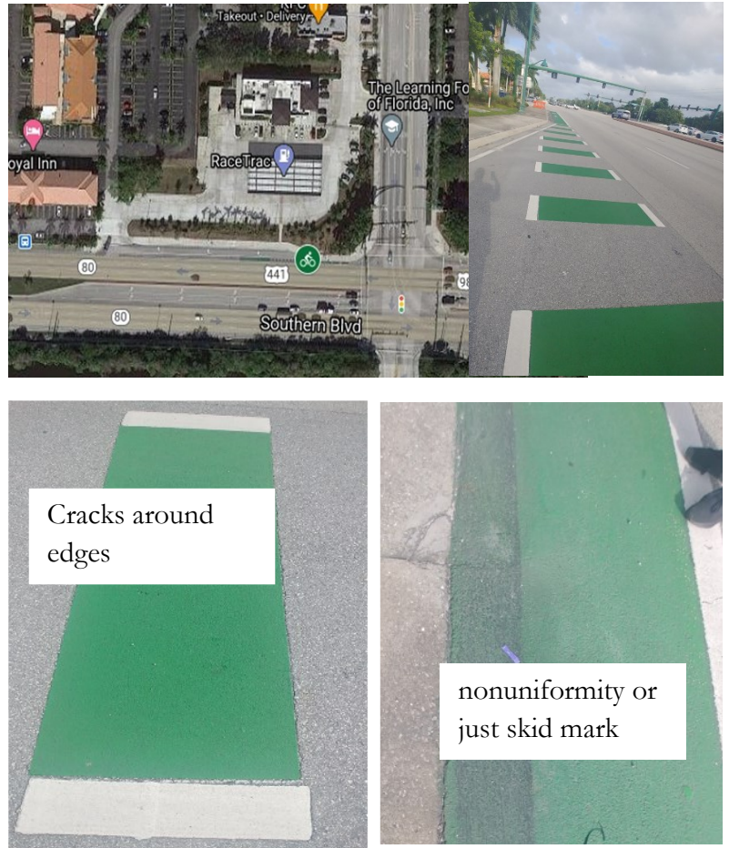
Figure A-17. Site 34-Location and Distresses.
