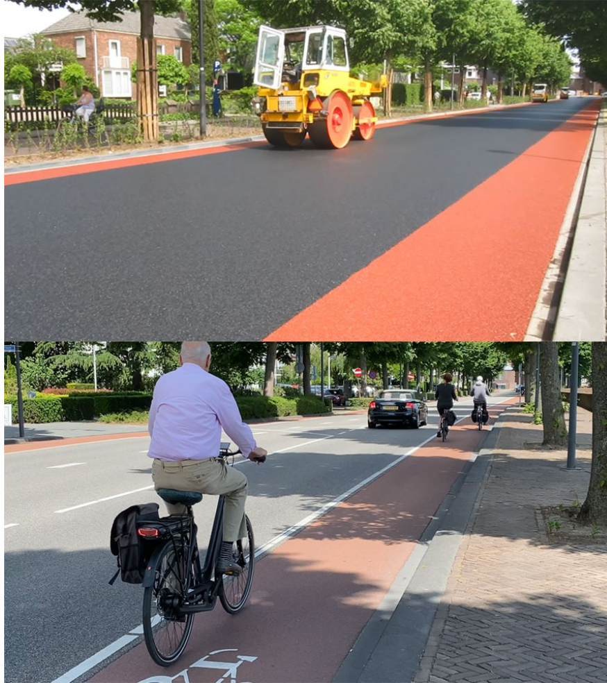
Figure 2-6. Colored Asphalt Bike Lane: New and Nine Years Old.
