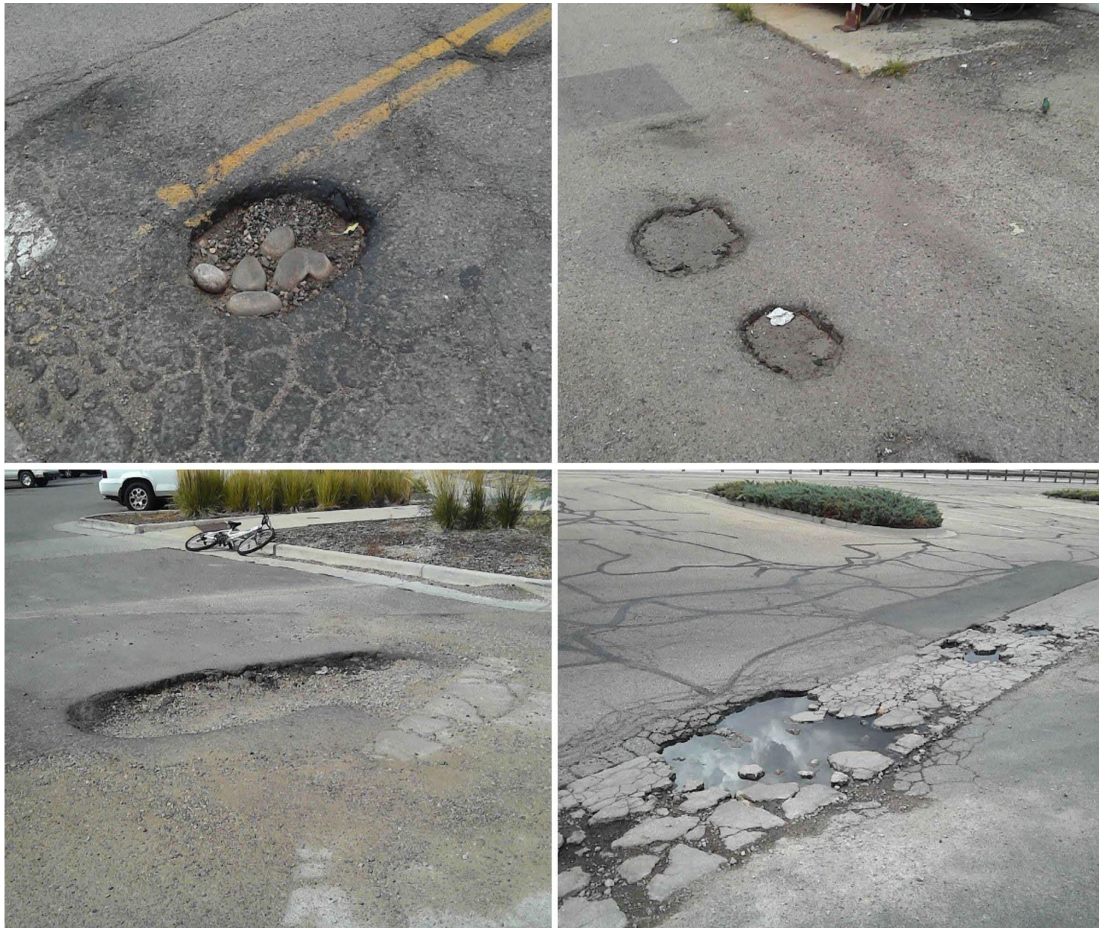
Figure 1.1 Samples of potholes
