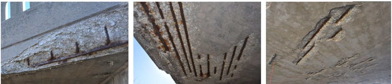
C. Close-up of damage
