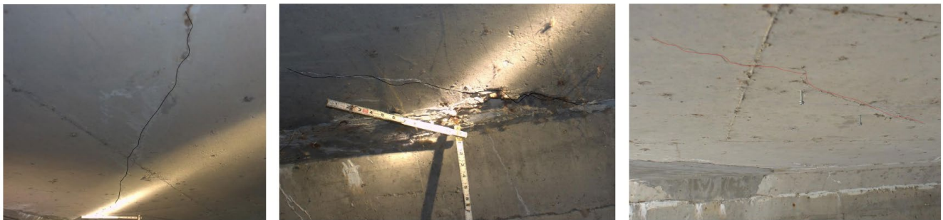
D. Localized damage
