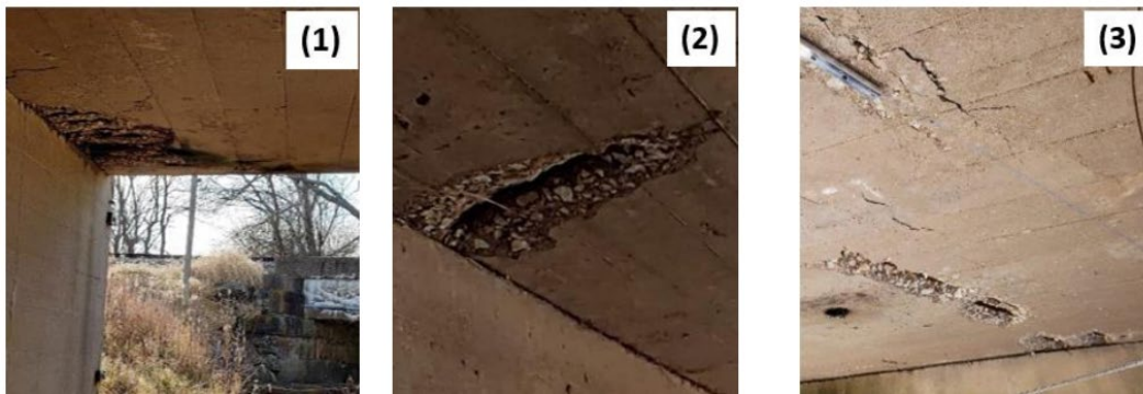
C. Photographs of the damage
