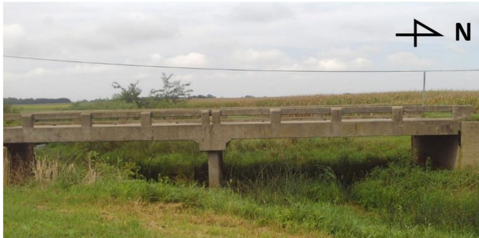
Figure 24. Photo. McLean County bridge.
