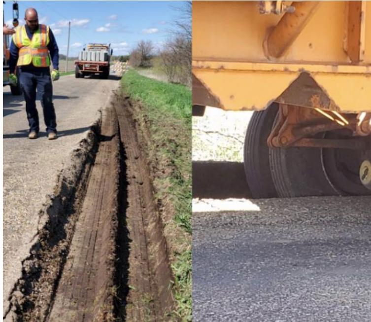
Figure 31. Photo. Damage to the road due to heavy axle loads during the proof load test of McLean County bridge.
