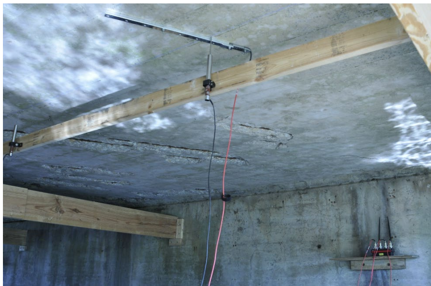
Figure 66. Photo. Photo of instruments under 0740016 bridge.
