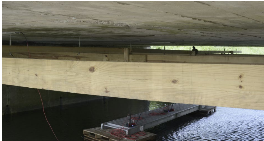
Figure 60. Photo. Photo of instruments under 0740013 bridge.
