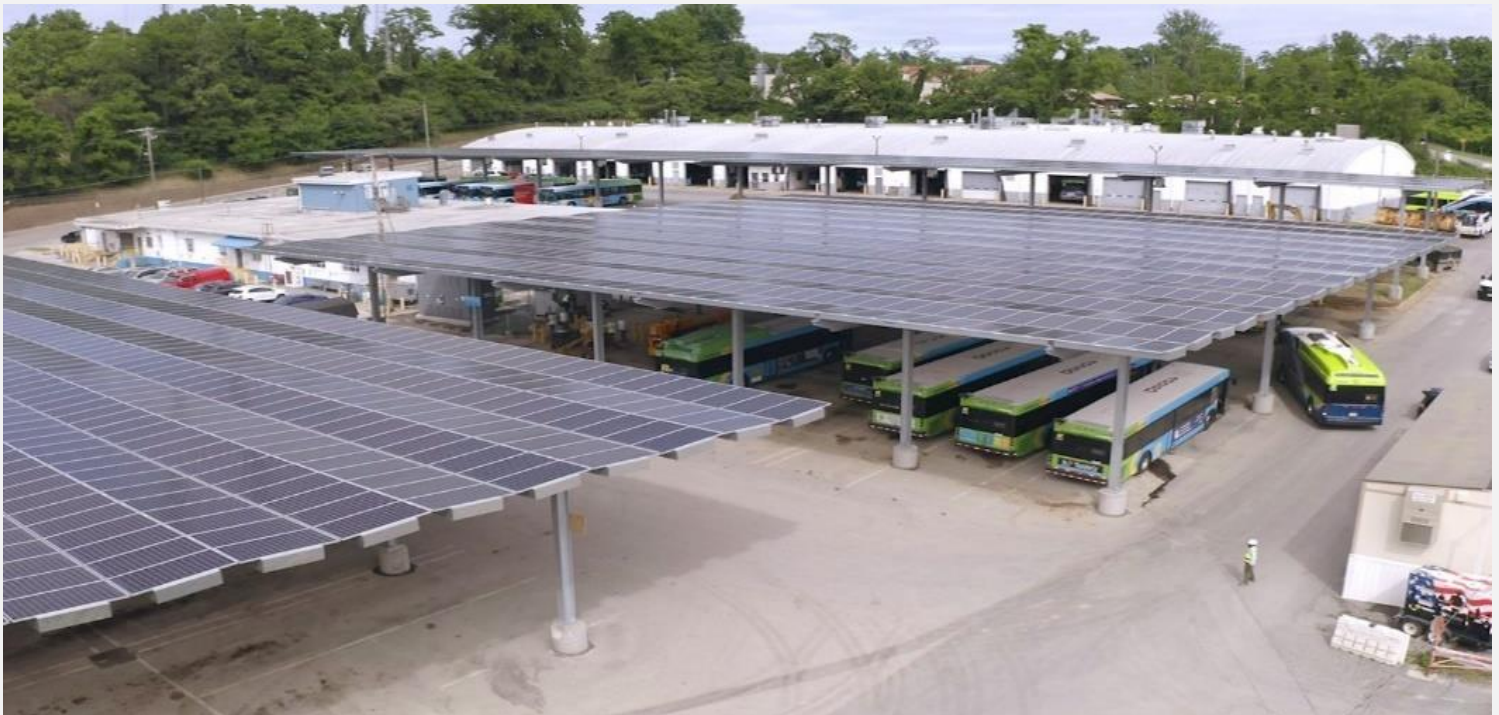
Solar Panel - 3D Canopy Source Montgomery County
