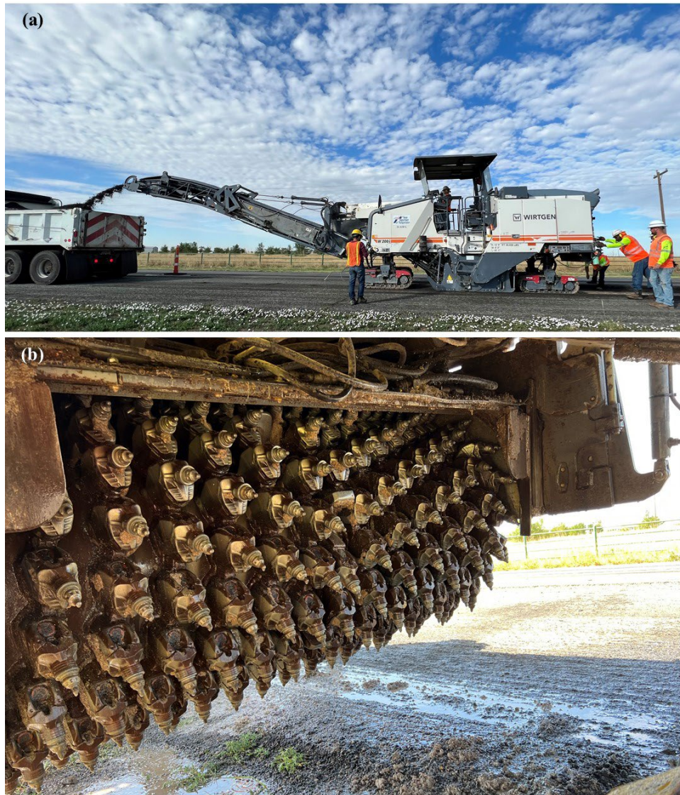
Figure 9.2. Milling operation to collect RAP and GRAP samples: (a) view of equipment during operations; and (b) detail of milling drum.
