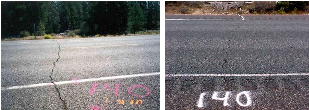
Figure 2.23. Photographic comparison of crack 140 before overlay construction (left) and reflection of crack through overlay after construction (right) (OR-RD-08-01).
