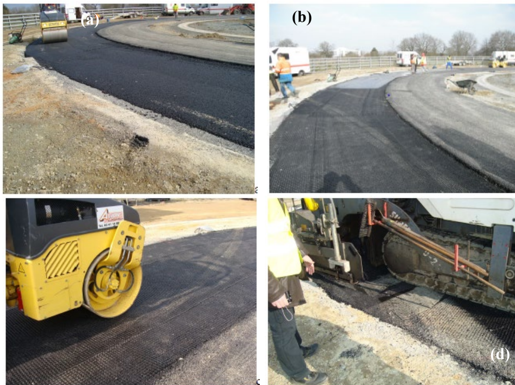
Figure 2.27. Photographs showing: (a) construction of 20-mm-thick bituminous layer; (b) fiberglass grid installation; (c) compaction of grid; and (d) paving of 50-mm-thick bituminous layer (IFSTTAR, 2012).
