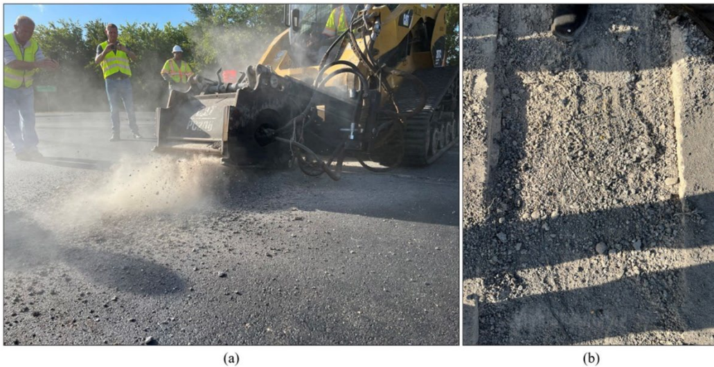
Figure 9.14. Milling of asphalt layer that had polyester (PET) geogrid: (a) milling operation performed at site; and (b) presence of PET geogrid fibers at the site.
