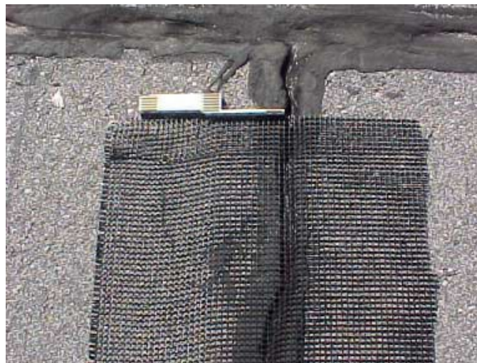
Figure 2.20. Photograph showing close-up of glass grid installed on a transverse crack (ME 01-3).
