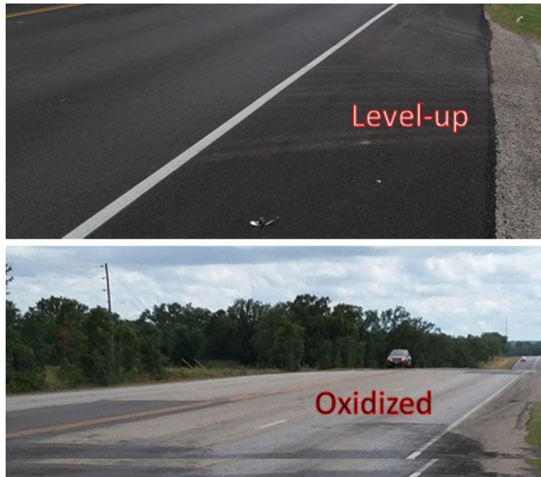
Figure 3.8. Asphalt surface condition: (a) level-up; and (b) oxidized.
