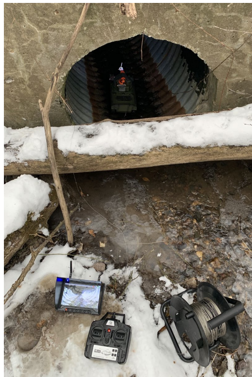
Figure 17 Mobility testing of HIVE 2.0 Tank in metal lined culvert with flowing water and separation gap in Culvert 64099 under U.S. Route 7 in Charlotte, VT
