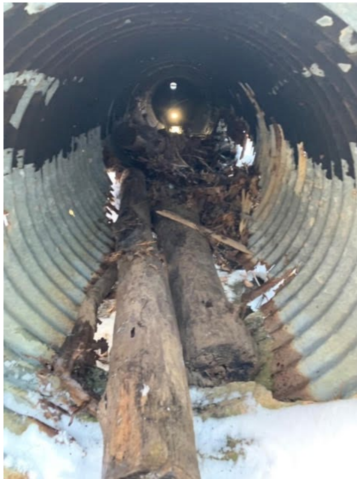
Figure 41 HIVE 1.0 stuck in separation gap of Culvert 64099, vehicle headlamp is visible.
