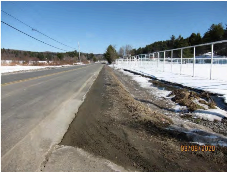
(b) V12A Roxbury-Northfield at Roxbury village (edge heaving on March 8, 2020)
