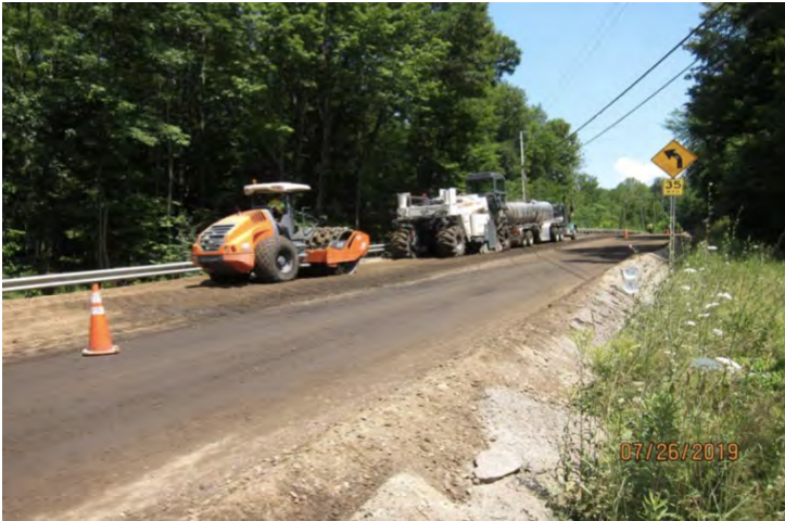
(a) Equipment train with grinder/mixer supplied by tanker truck and followed by sheep's foot compactor
