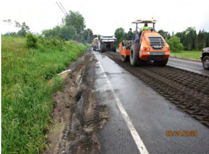
Equipment train with reclaim grinder/mixer supplied by water tanker truck with sheep's foot compactor behind
