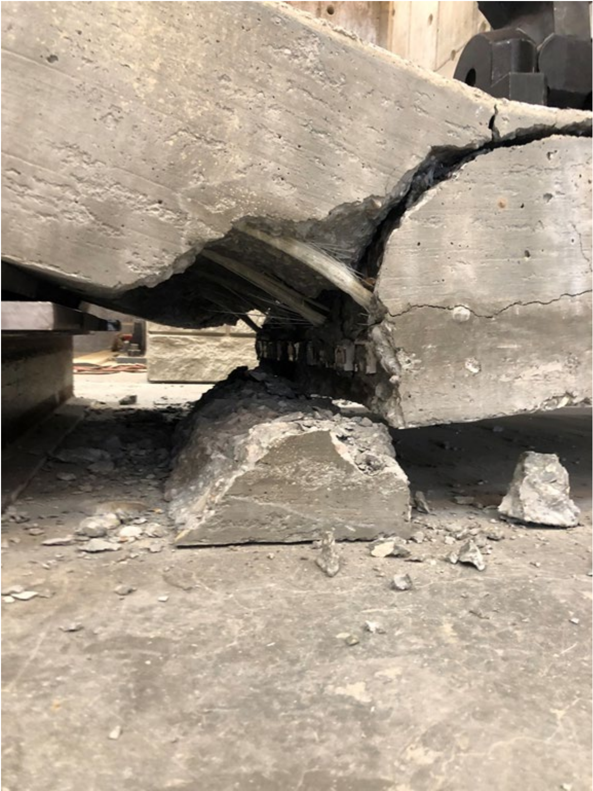
Figure 5.21 GFRP Reinforcement Failure
