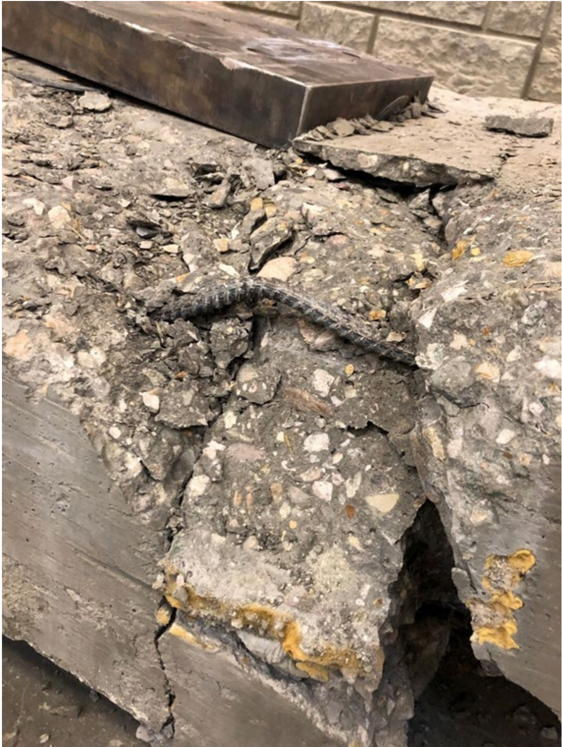
Figure 5.11 Steel Reinforcement Failure
