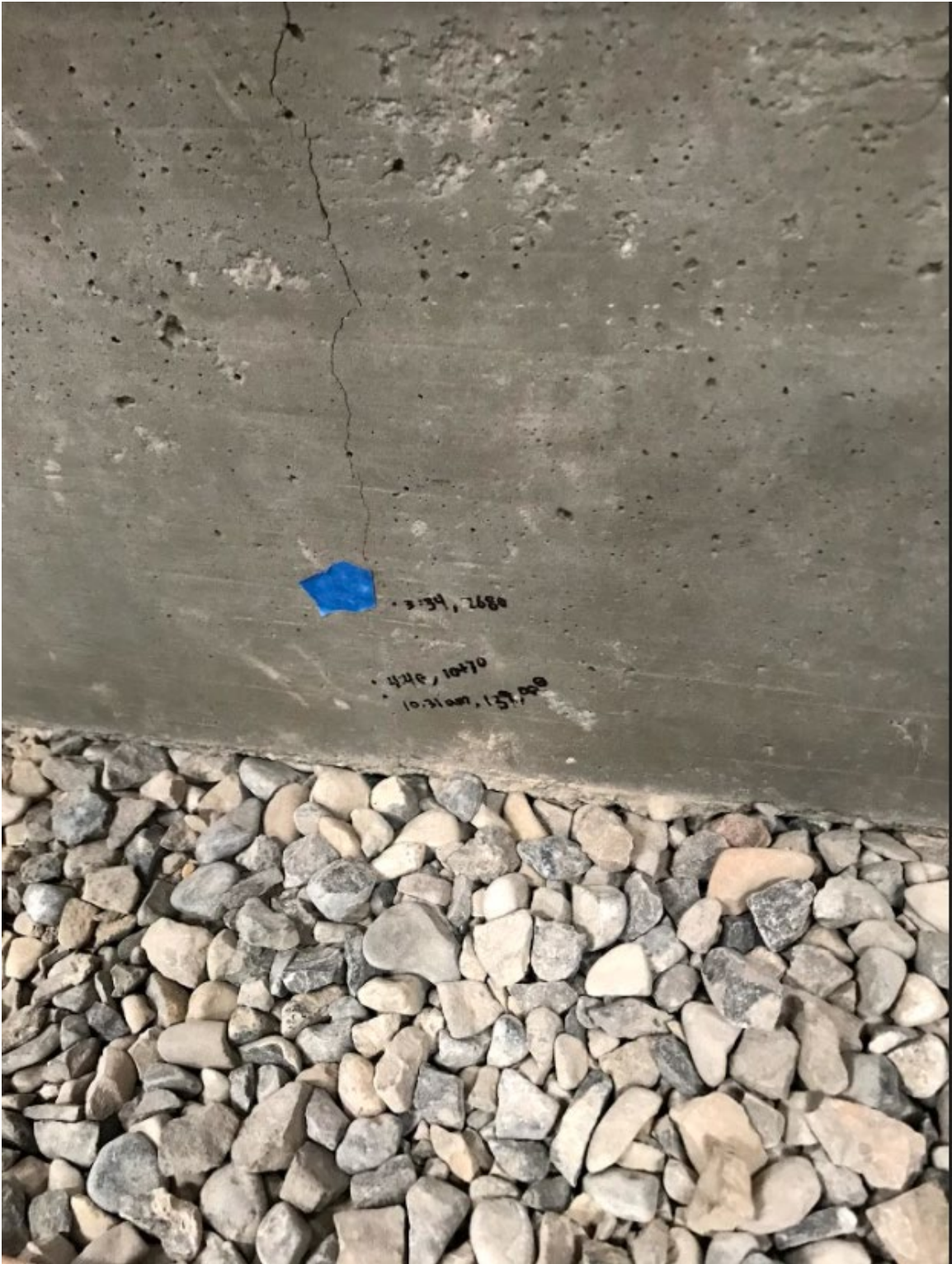
Figure 5.16 GFRP Side Cracking
