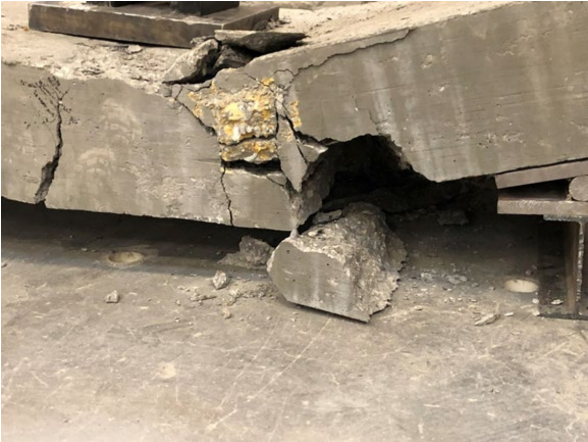
Figure 5.9 Spalling Slab with Steel Reinforcement
