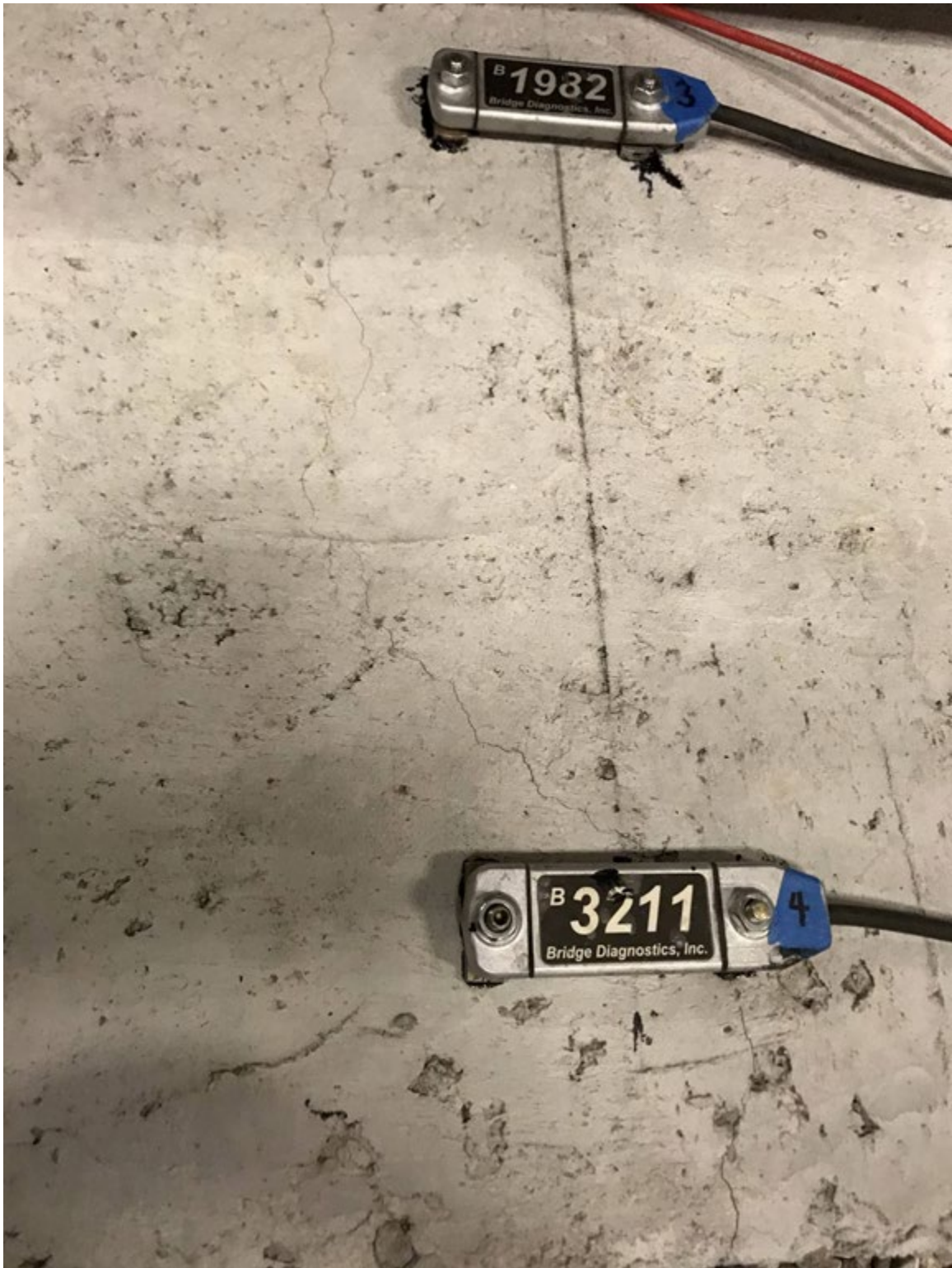
Figure 5.15 GFRP Surface Cracking
