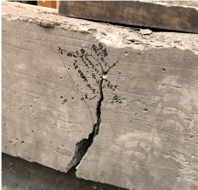
Figure 5.5 Steel Cracks at Failure
