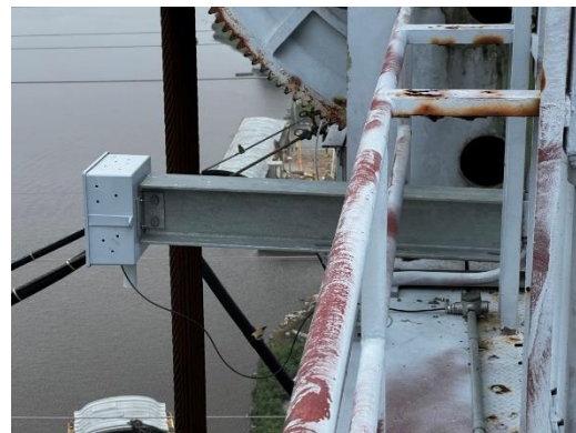
(b) Final laser installation at NW location
