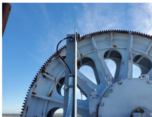
(b) Inclinometer wireless antenna at north tower
