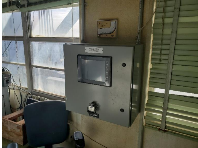
Figure 11. Operator’s main SMART relay HMI and skew enclosure
