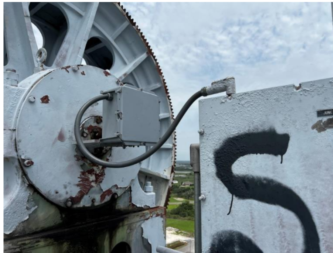
Figure 3. Southwest encoder final installation with cover
