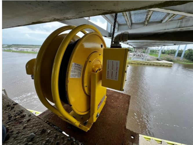
Figure 17. Cable reel used in attempted Power Line Communication
